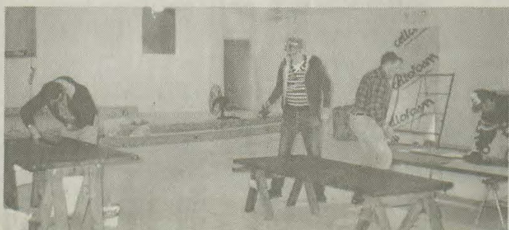
In photo to the left, pastor Randy Orsborne (left), Floyd Daniels (center), James Allen, and Don Hughes stained church doors.
