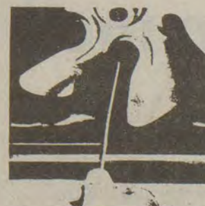
Water collected under the fan is a sure sign that the drain hole is clogged. Push a stiff wire, such as a straightened-out clothes hanger, down the drain hole to remove any debris that is clogging it.
