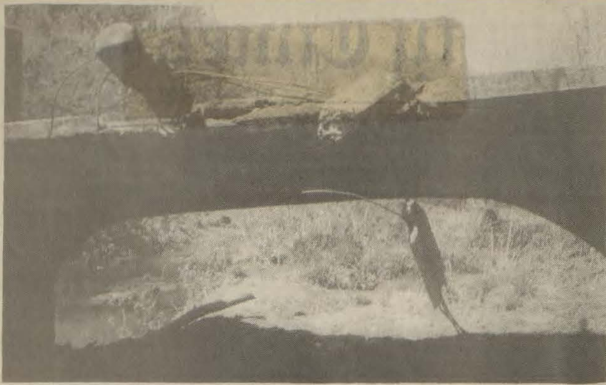
'Hunter Bridge Is Falling Down'
