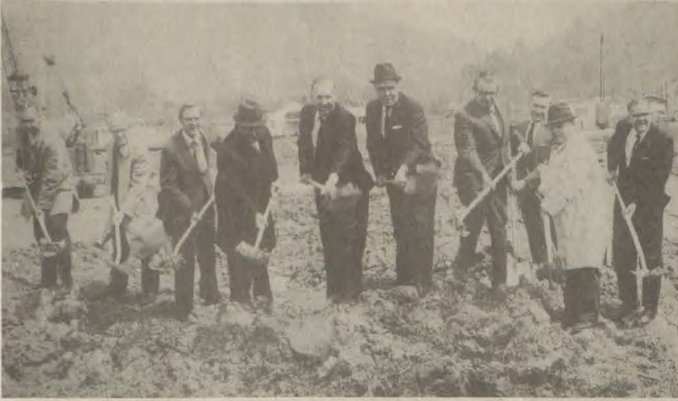
It was April 4, 1970 when ground was broken, paving the way for construction of Highlands Regional Medical Center. On hand for the ceremony and wielding shovels were, from left: Allan Perry, Burl Spurlock, James N. Grey, Russell Williamson, Congressman Carl Perkins, Dr. George P. Archer, James Carpenter, Robert Nolan, Harry LaViers, and Chalmer H. Frazier. Highlands is celebrating its 15th anniversary this year.
