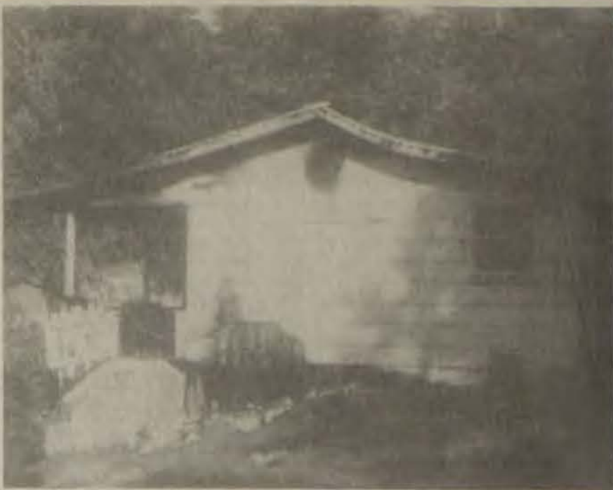
(Photo by Allen Bolling) FOLLOWING A FIRE, Monday, at West Prestonsburg, the walls of this frame house were still standing, but Prestonsburg fire fighters said the structure was "well gutted" by flames. Arson is suspected in the incident.
