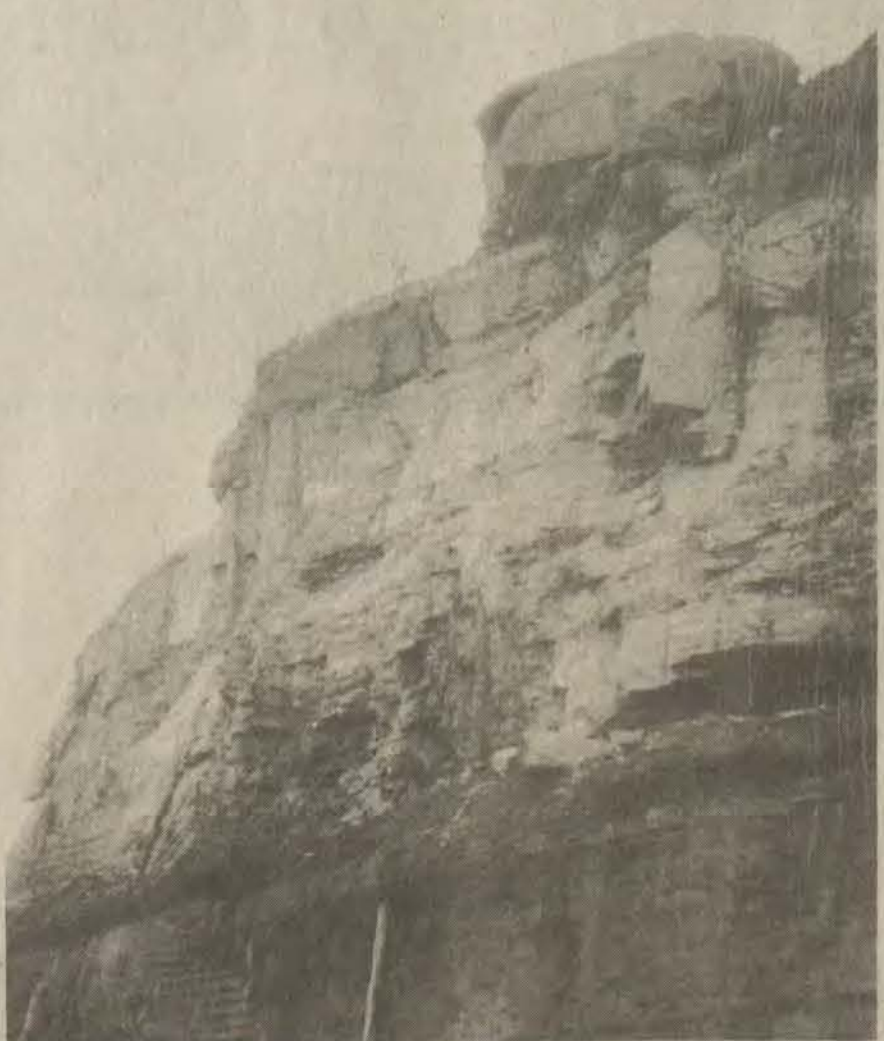
A HUGE BOULDER which threatened to fall from a highwall at Prestonsburg Village Shopping Center was successfully repositioned, Friday, as it teetered on the edge of a coal seam. The work forced the evacuation of Winn-Dixie's, Wal-Mart and McDonald's.
