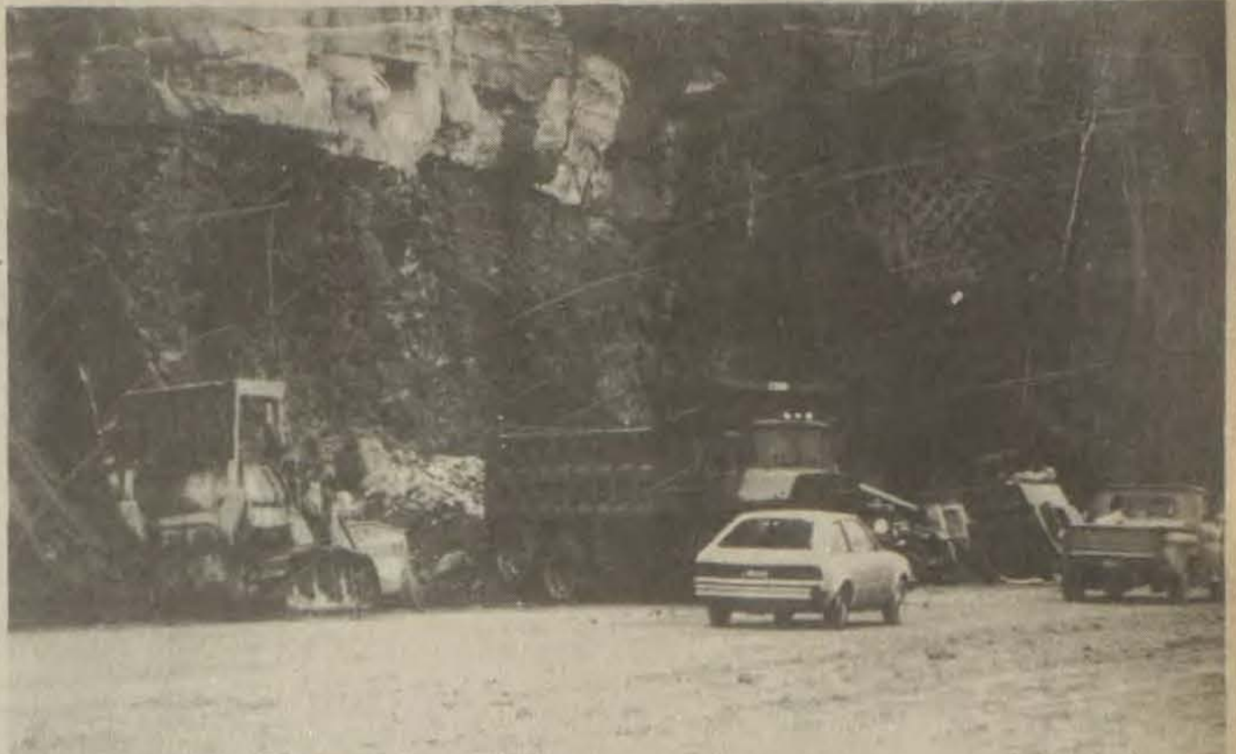
PREVENTIVE MEASURES were taken on US 23 between here and Paintsville, this week, as highway department members blasted dangerously loose rock from the near-perpendicular cuts in a hillside bordering the road. This is being done to avert the rock falls which plague the road and its travelers.
