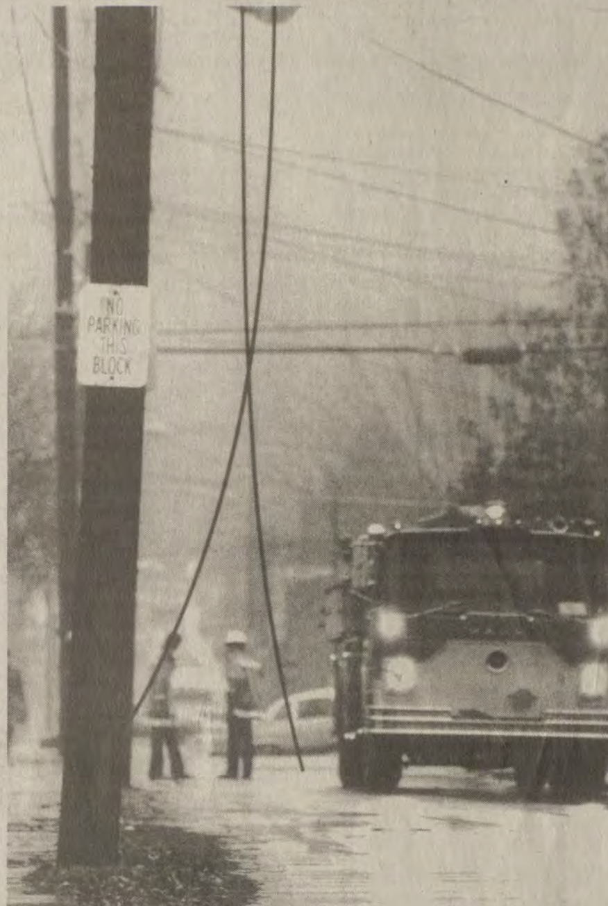
THESE DANGLING WIRES pulled loose from an insulator caused an hours-long power outage, here, Monday afternoon.
