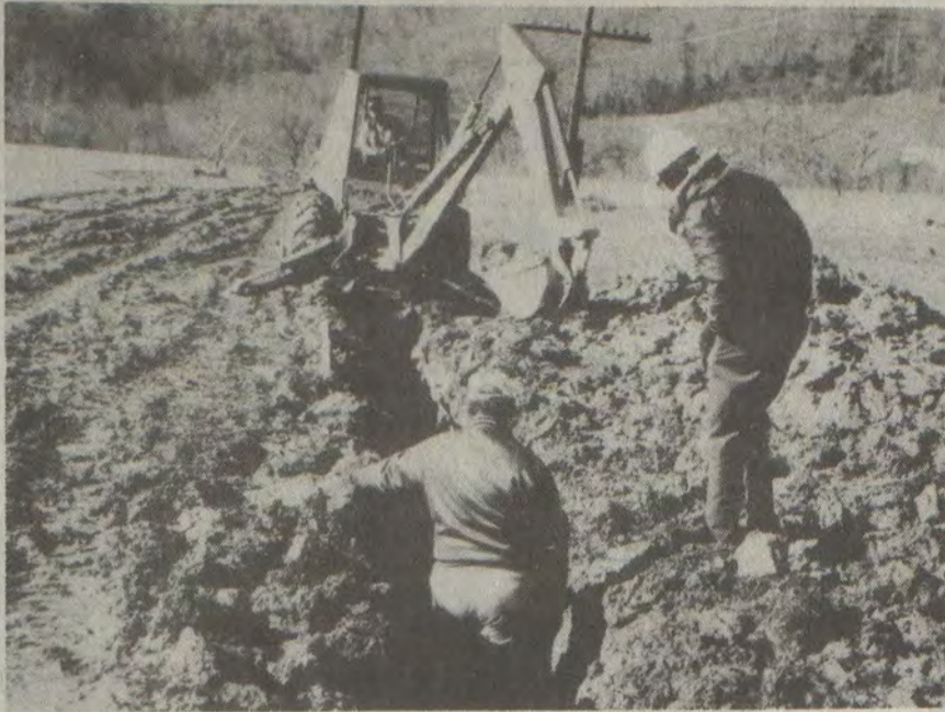
During construction of a drainage ditch, Oscar Rice and Clark Allison check progress for backhoe operator Troy Jarrell. This job was done at the John M. Stumbo Park at Allen, in preparation for a total renovation of the golf course later this year.
