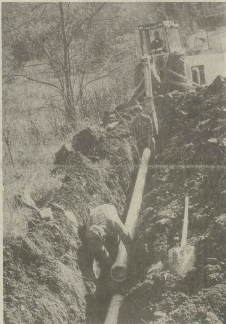
WATER MAIN destined to serve 323 Prater Creek families was being laid Monday at the mouth of Rice Branch. Lowering the six-inch pipe into a trench dug by Lonnie Jordan was Johnny Robinson, foreground, and Keith Wolfe. The Greenup county men are employed by Claud Wilburn and Sons, of Maloneton, chief contractor for the $1 million water system.
