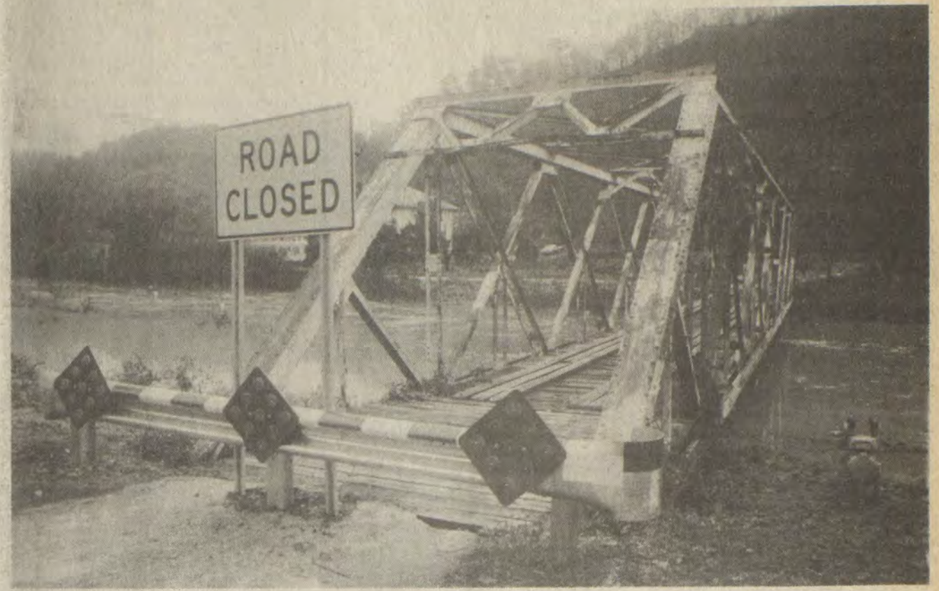
THEIR WAY BARRED by order of federal highway authorities, Glo residents were organizing last week to get the bridge serving their community repaired and reopened. Access for 32 families in the old coal camp is also available via Estill and Wayland, but over roads the residents say are dangerous and out of the way.
