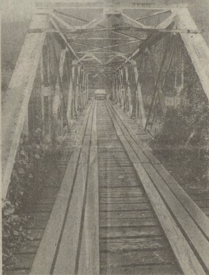
THE FLOORING was recently repaired but the steel structure of this bridge at Glo, which residents say predates the advent of motorized traffic, has so deteriorated the bridge should be closed until it is replaced, according to state Transportation Cabinet officials. The bridge, which serves 26 families in this Right Beaver community, remains open, but Floyd Fiscal Court recently authorized Judge-Executive John M. Stumbo to negotiate with the state for help in replacing the structure.
