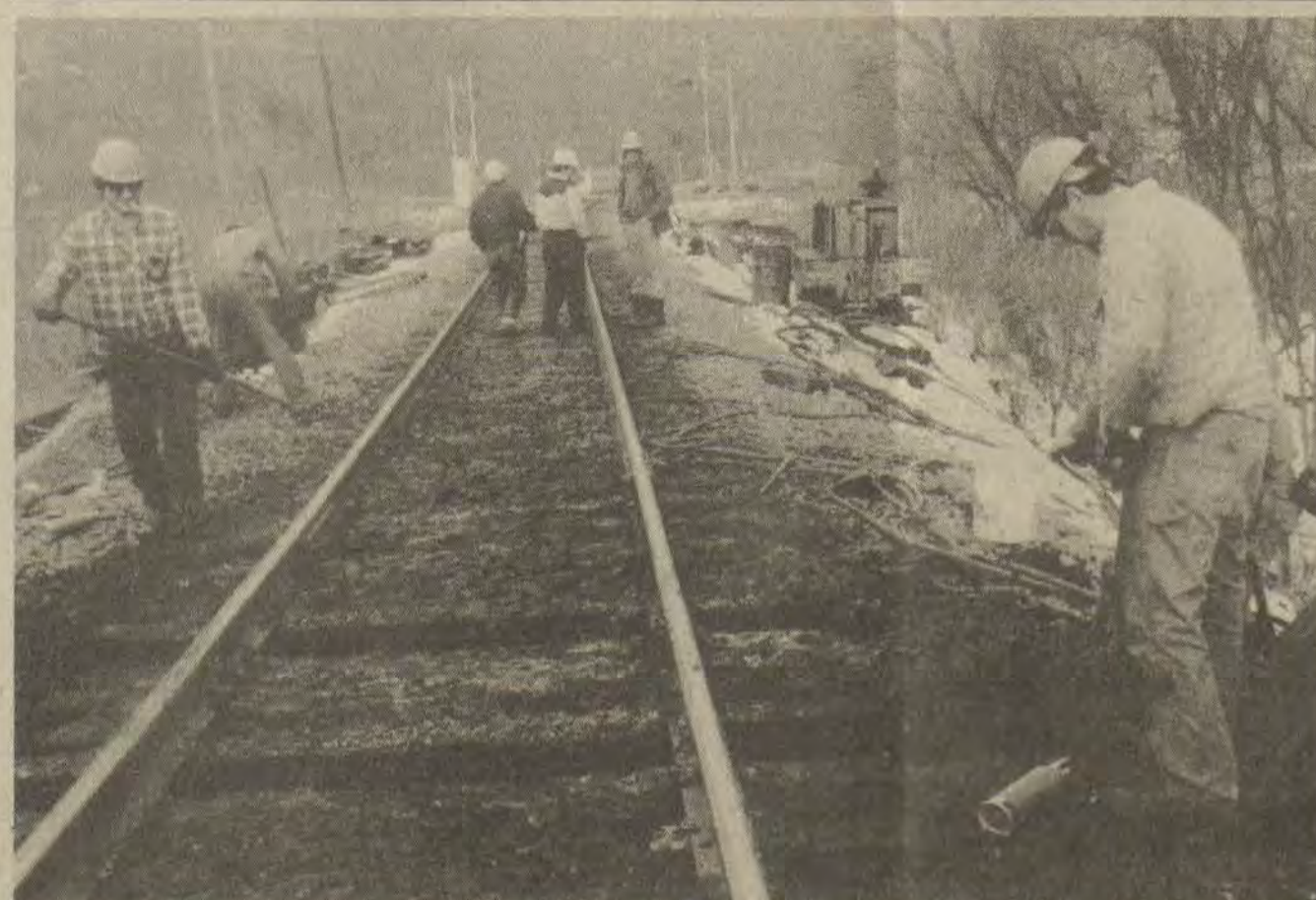
WEATHER PERMITTING , which hasn't been too often lately, railroad crews have been out doing maintenance and light construction. Here C.&O. workmen are shown preparing to renovate a bridge abutment near the Goble-Roberts Addition.
