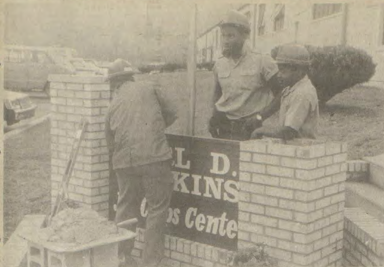
JOB CORPS STUDENTS erect a new sign outside the center here displaying its new name—The Carl D. Perkins Job Corps Center. The center was renamed in the late congressman's honor during ceremonies last month.
