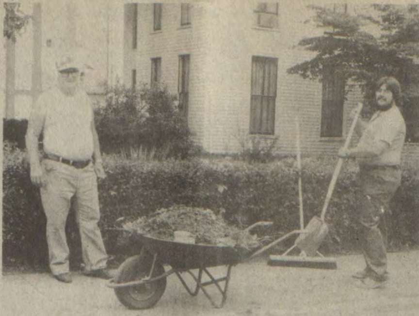
SIDEWALKS HERE ARE LOOKING SPRUCER THIS WEEK as city workmen wield shovels, brooms, and yes, a good old-fashioned wheelbarrow to collect accumulated debris.
