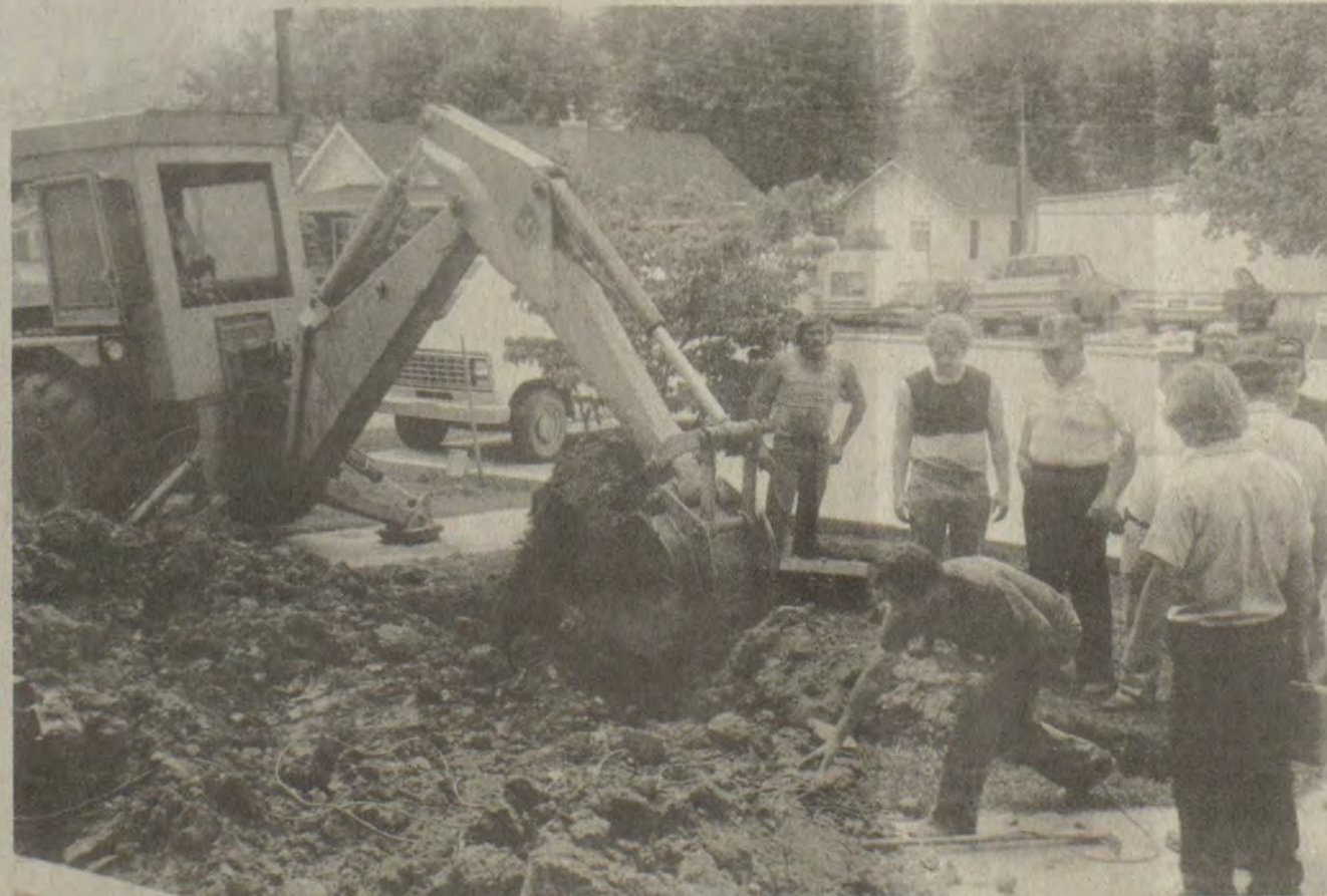
THE NORMALLY-BUSY courthouse stood deserted and malodorous in Prestonsburg this week as sewage backed up and entered first-floor offices—the handiwork, it was said, of some inmates in the third-floor county jail. By feeding a wire into the sewage line, workers with the Royal Flush Rooter Service were able to retrieve sheets and bedding from the line. Some offices may be closed for several more days, courthouse officials said.
