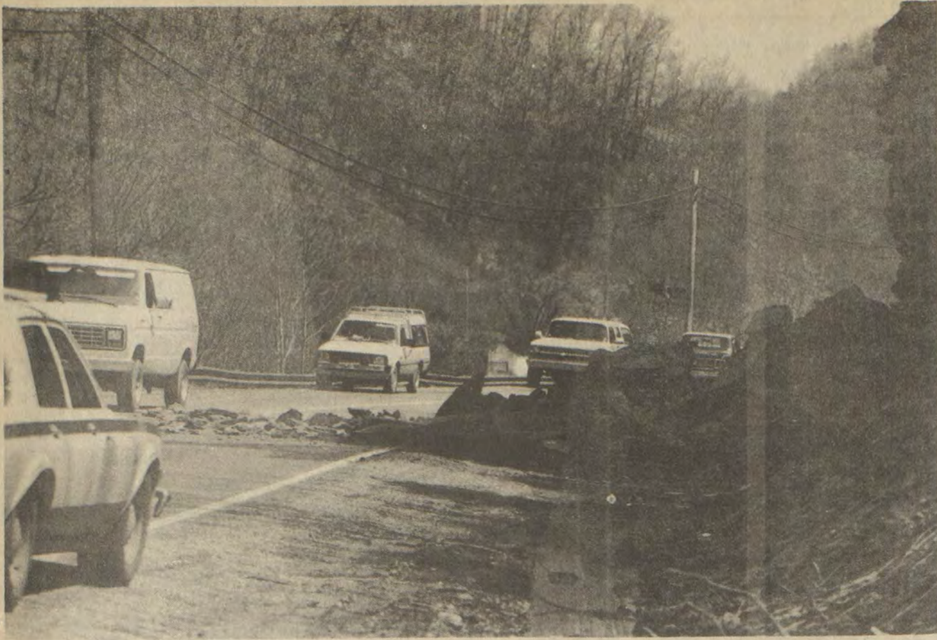
MAYBE IT WAS ALL THE RAIN, or the unstable nature of the shale and decomposing sandstone which form the cliffs along U.S. 23. Certainly the design of the road cuts which ignore any sort of terracing played a part. But whatever the reason, a recent rockfall from the cliff just north of the college here blocked traffic for a time and occupied road crews for several hours. Such slides are common and make the heavily-travelled route one of the more risky stretches of highway around.
