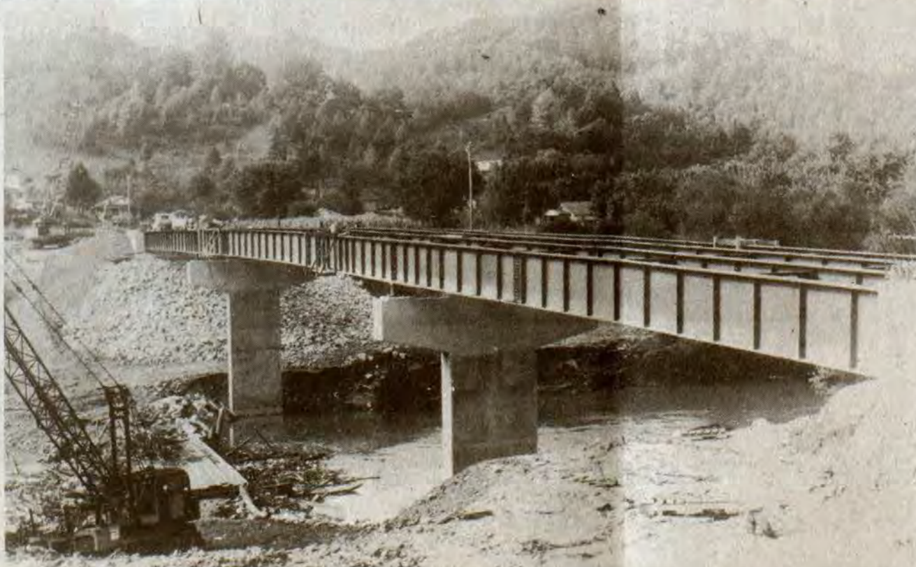
SPANNING THE BIG SANDY at Tram, girders of the new bridge there were recently lowered into position. Construction costs for the bridge, which is being erected just downstream from the rickety suspension bridge it will replace, were estimated at $888,000 by the state Department of Transportation last year. The bridge is being built by Kay and Kay Construction, a London firm.
