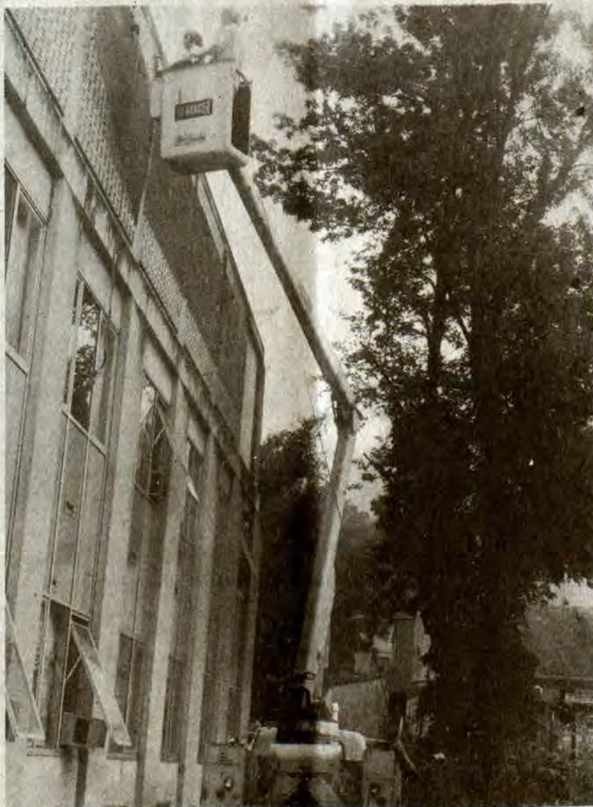
INSTALLATION OF WIRE shielding over jail windows will, when complete, deny some prisoners a favorite pastime—letting a line down to the ground where a relative or friend waited to attach to it a packet of marijuana or other contraband.
