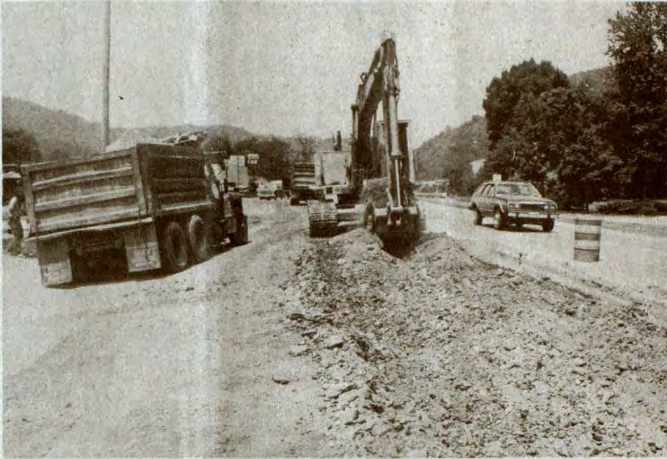
ALTHOUGH A TEMPORARY INCONVENIENCE, motorists in the Prestonsburg area will eventually be rewarded with a more permanent improvement of access and traffic flow in the congested section of U.S. 23 from near the Pic-Pac Supermarket to Prestonsburg Community College when work by the state Department of Transportation has completed widening of that stretch of highway. The project, attained largely through efforts of the Prestonsburg City Council, is being accomplished through state Road Improvement Funds totalling $240,955.
