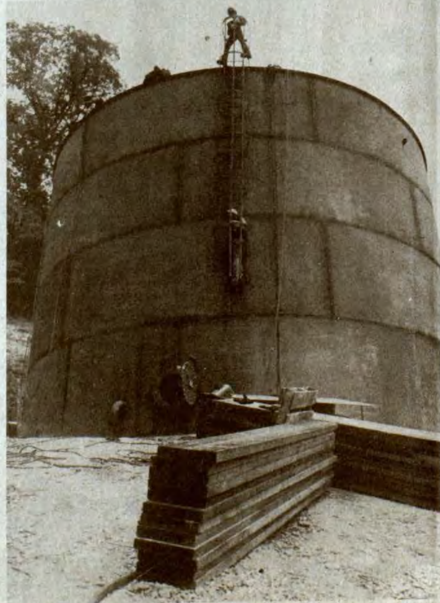
CONSTRUCTION of a 310,000-gallon water tank at Allen, shown here in progress, is part of the Prestonsburg water system's $4.2 million dollar expansion project. Caldwell Tanks, of Louisville is contractor on the work at Allen.
