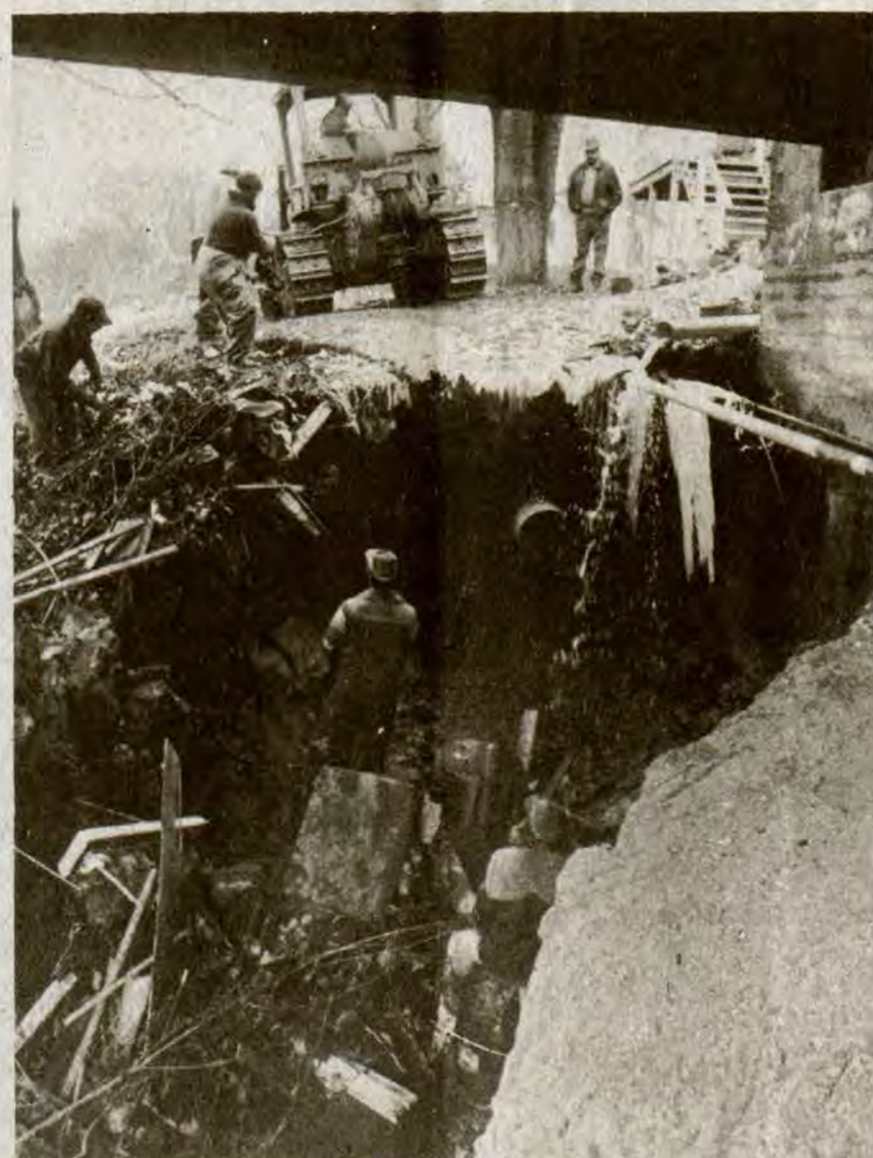
WATER OFFICIALS and workmen survey conditions following the rupture, Monday night, of a Beaver-Elkhorn Water District line at Martin which left 1300 customers of the system without water and caused considerable erosional damage beneath the bridge which crosses Beaver Creek to Buck's Branch. A line of the Martin water system, said to be within 20 feet of the Beaver-Elkhorn pipe, also burst the same night in a discouraging coincidence, cutting off water to Martin residents.
