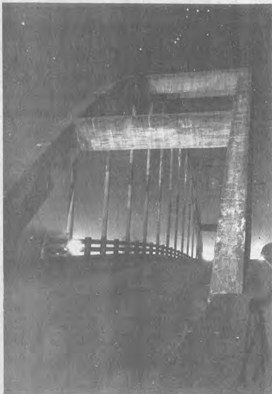
THE WEST PRESTONSBURG BRIDGE, pictured here aglow on a recent moonlit night, has been closed to traffic for several years, but with its unusual architectural styling, it remains a landmark in the Prestonsburg area.
