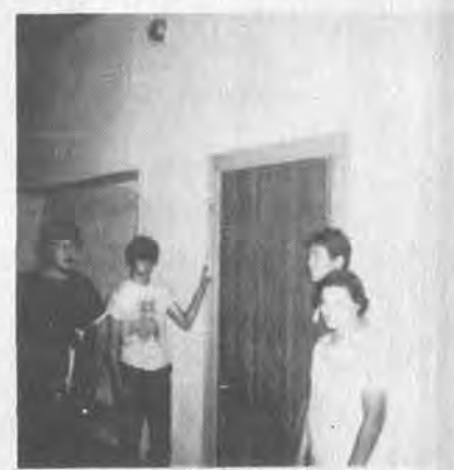
Installing paneling on either side of doors for reinforcement to meet fire standards. As a result of work by SYEP Participants, Garrett School received a 1R-Rating according to Fire Standards.
