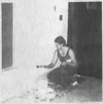
the quality of paint, proper blend in mixing paints, compatible colors and color schemes. A total of 1,342 gallons of paint was used by SYEP Participants in renovating nineteen school plants.
