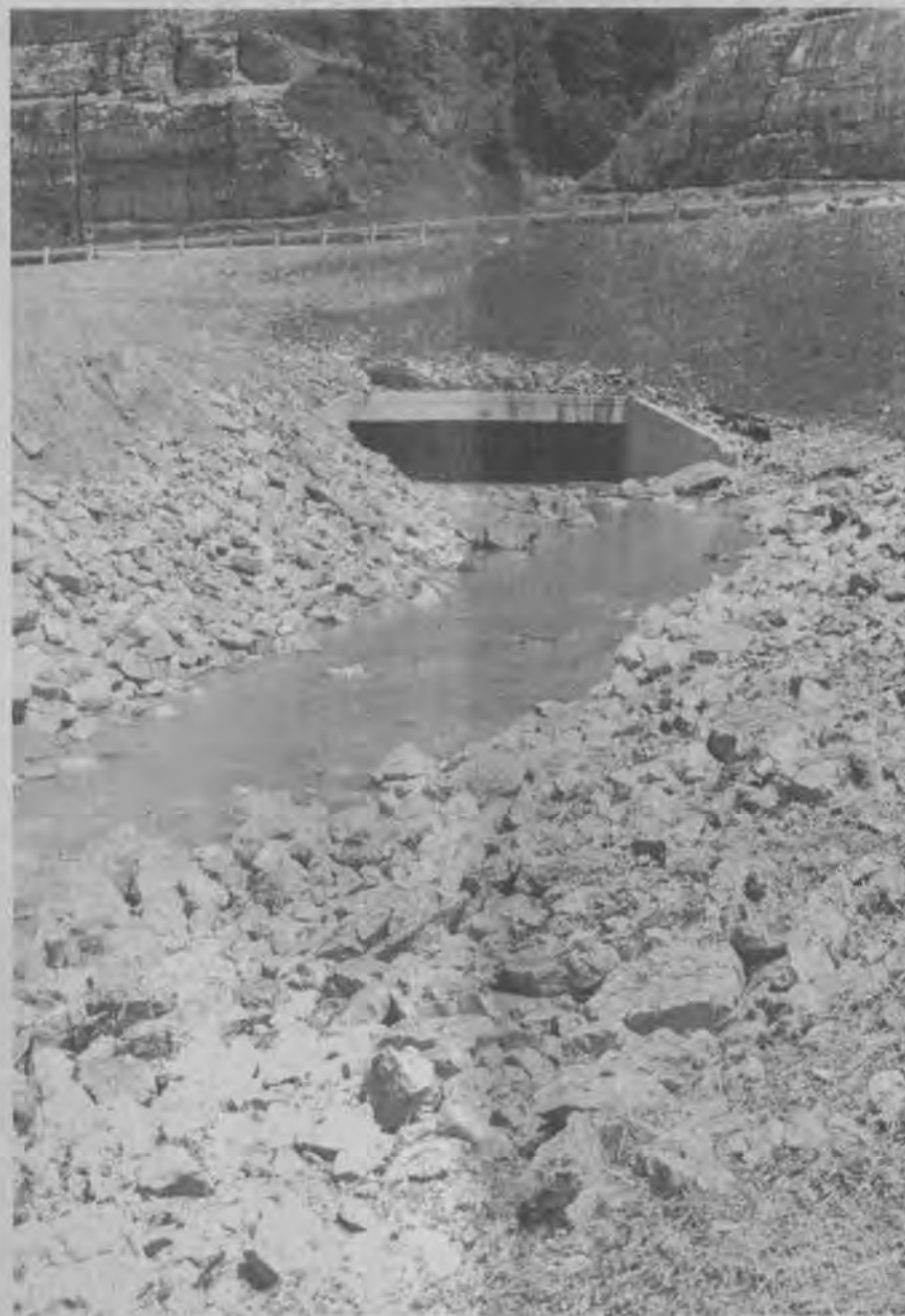
FILLS AND CULVERTS, created by the construction of new KY 80 on Rock Fork near Garrett contributed to severe flooding along the creek following heavy rains over the weekend of June 6, according to many residents of that section. They contend that the culvert openings are too small to handle runoff while the fills act as dams.
