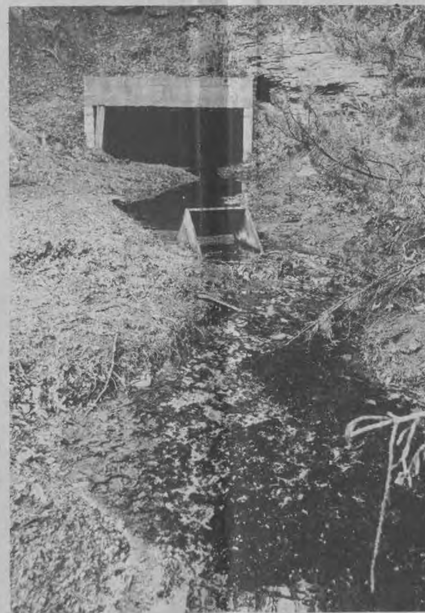
ACID WATER flows from the mouth of an abandoned mine on Rough and Tough Branch at David, one of four along the hollow which have for years rendered the entire length of the left fork of Middle Creek incapable of supporting aquatic life. Stopping the runoff is a priority of work initiated last spring as part of the U. S. Department of Agriculture's Soil Conservation Service Rural Abandoned Mines Program.
