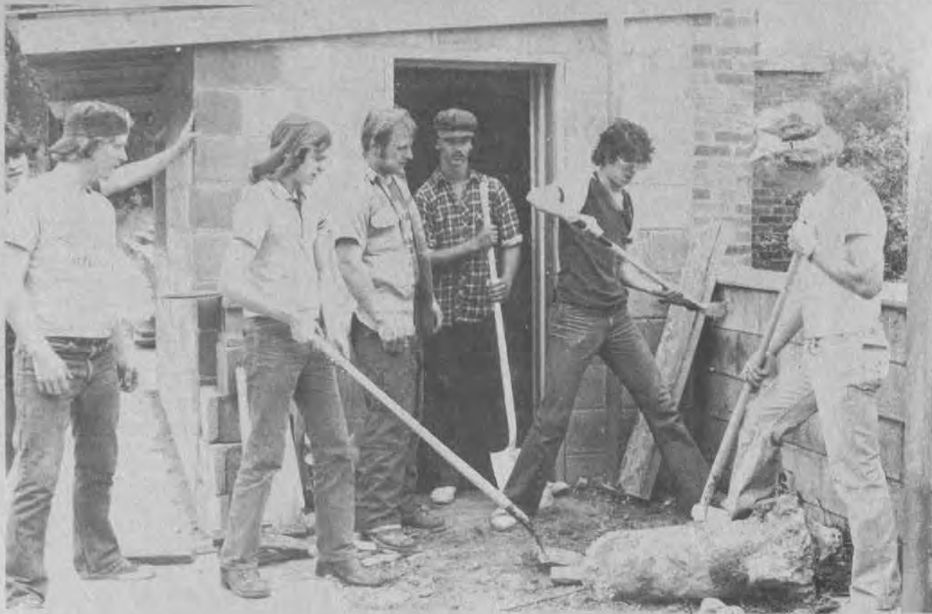
A JOB CORPS masonry class has nearly completed construction of a concession stand at the Archer Park softball field. The Corps is furnishing all labor for the job, which has taken about a month. The new concrete-block structure replaces a portable stand formerly in use at the field.
