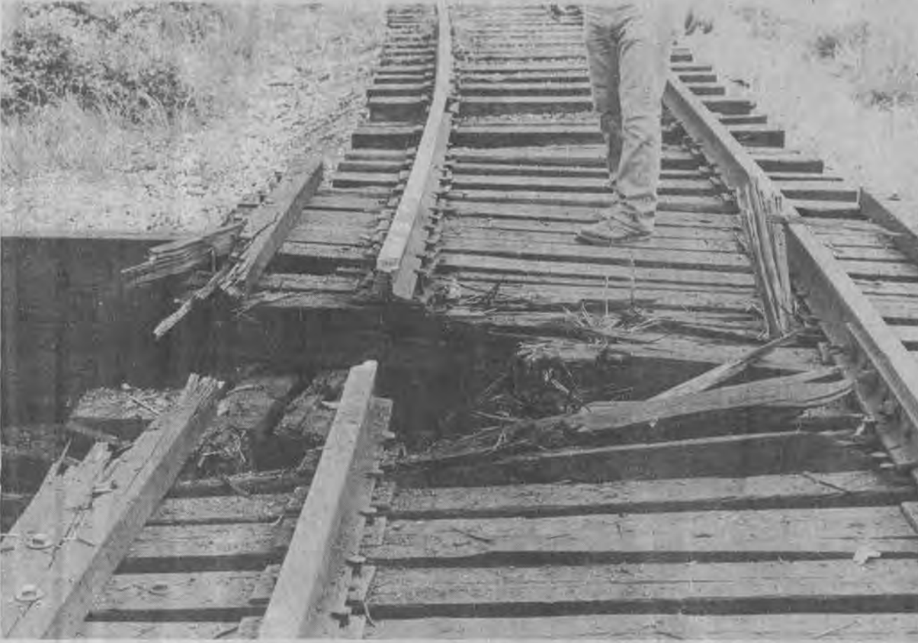
DAMAGE TO C. & O. railroad bridge near the junction of state routes 1210 and 404 on Middle Creek is shown in photo taken Tuesday morning. Cross-ties and heavy timbers were splintered and a section of rail was blown away by an explosion which occurred in the early morning hours, Tuesday. A second blast, Tuesday morning, also damaged a C. & O. bridge between Warco and Maytown. State and federal officers are investigating the incidents.
