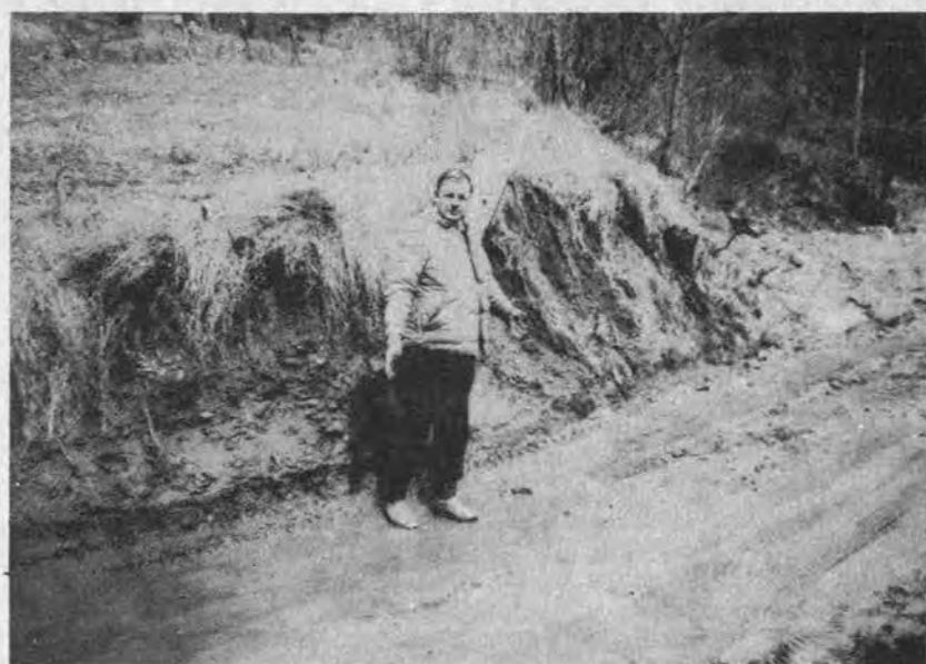
Ditchline needs work on Prater Creek road.
