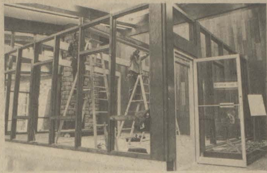
MAJOR RENOVATION WORK was begun in recent weeks at May Lodge, Jenny Wiley State Park, part of a planned $300,000 facelift for the park which is expected to be completed by next April. Photo shows work progressing on relocation and enlargement of the gift shop at the lodge.
