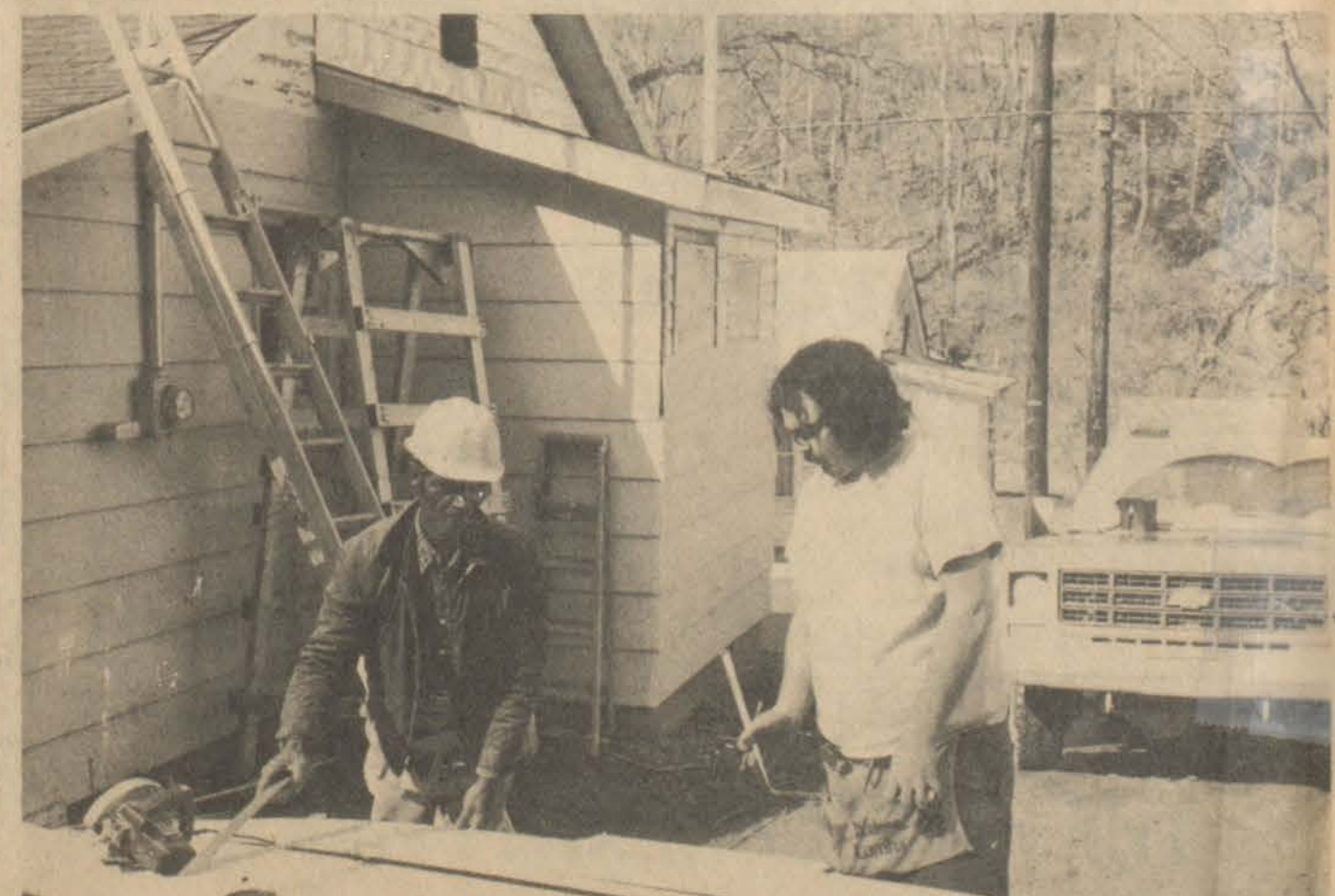
WORKMEN REPLACE SIDING on one of seven homes being renovated in Wheelwright's Branham's Hollow section last week. Thirty homes, owned by the Floyd County Community Development Agency, are scheduled for renovation and sale this year.
