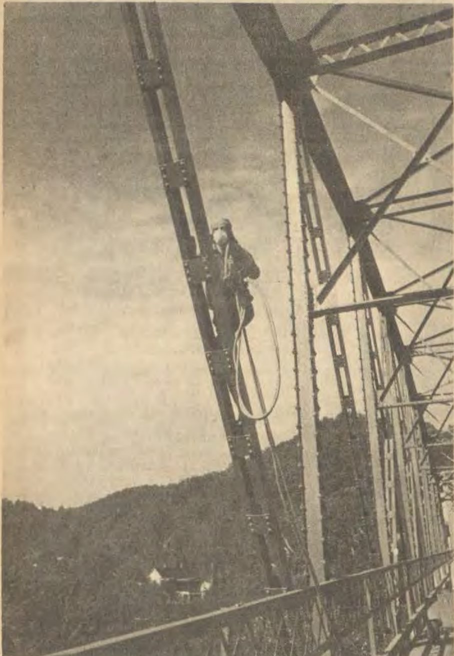
THE CLIFF BRIDGE received a coat of blue paint this week. Painter, pictured here in protective garb, is employed by the Panelis Corporation, of Youngstown, Ohio.
