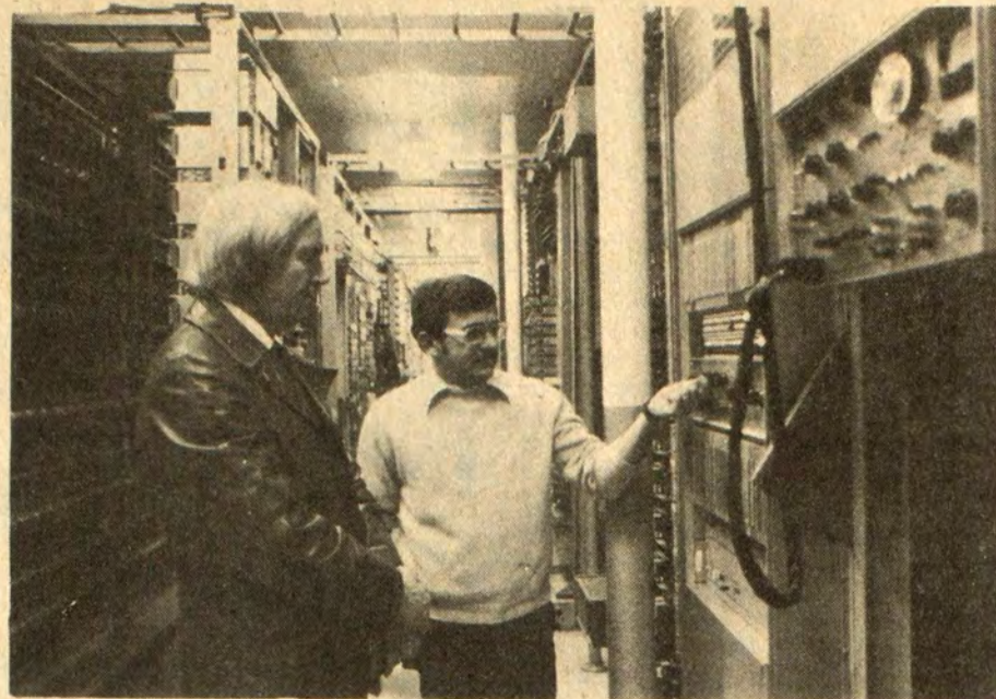
Bill Osborne, a South Central Bell supervisor, shows local Bell manager Phill Scott the mobile phone section of the new Prestonsburg telephone switching system. The new ESS begins service March 31.
