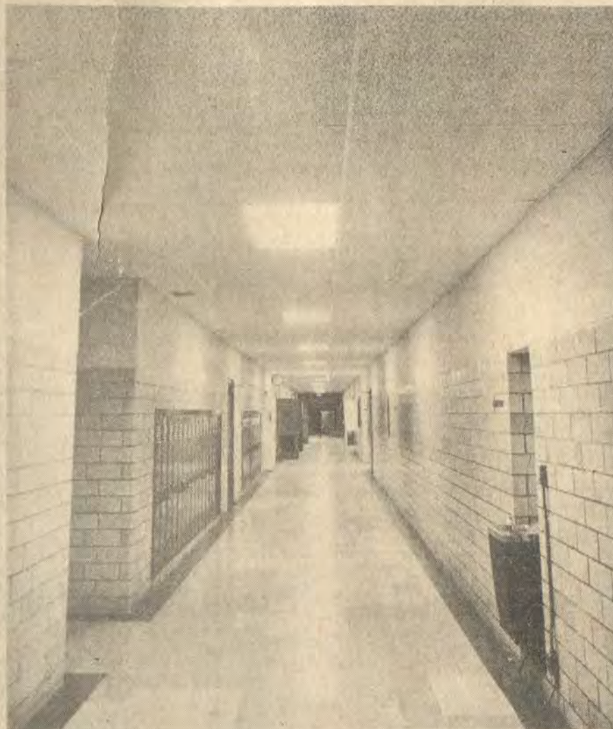
NEW CEILINGS at Prestonsburg High School replace the original heavy coating of asbestos which has been the object of removal work in recent weeks.
