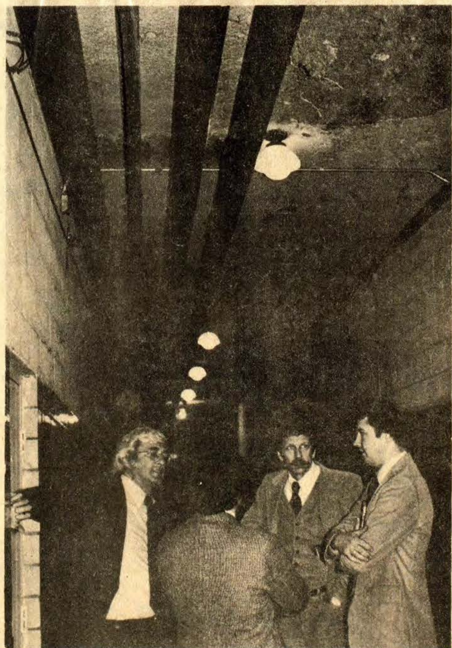
Pictured at last Tuesday's inspection of the widely publicized asbestos situation at Prestonsburg High School are, from left, Dr. Robert M. Sawyer, Yale University consultant on asbestos; Larry Dorsey, U.S. Environmental Protection Agency (EPA) representative; Jack Wilson, representative of the state Department for Natural Resources and Environmental Protection, and Jack Hyde, OSHA specialist who conducted original testing to determine asbestos concentrations in air samples from PHS.
