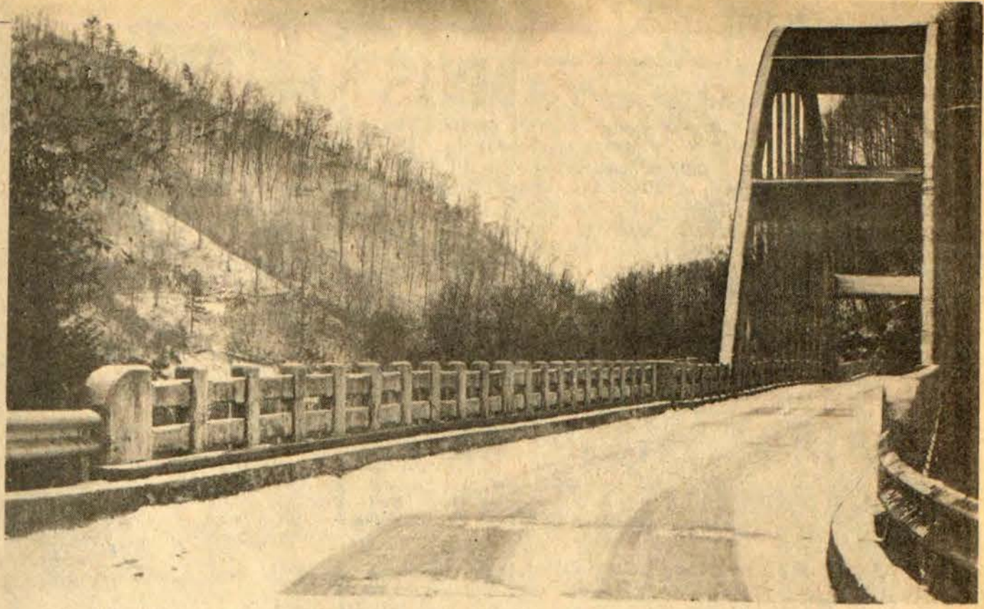
SNOW, SUNDAY NIGHT made for slippery driving through much of Monday along sideroads and especially on bridges resulting in the cancellation of classes in Floyd county both Monday and Tuesday. Pictured above is the icy surface of the Town Branch bridge here. Most county residents were glad to see the snowfall, however, as it slowed the rise of swollen area streams.
