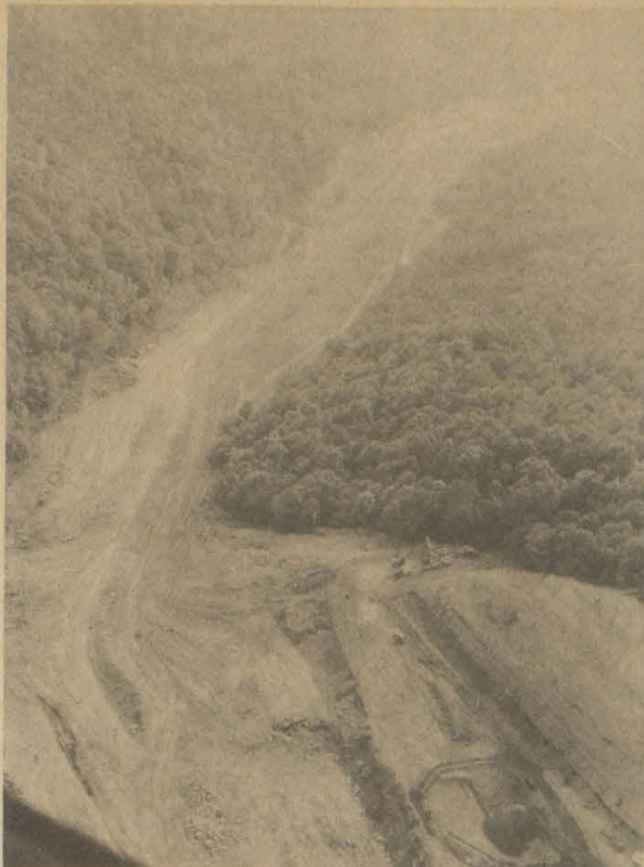
Aerial photo by Arley Hayes shows mountain top cut-through between Goose Creek and Garrett Hollow in the construction of new KY 80.
