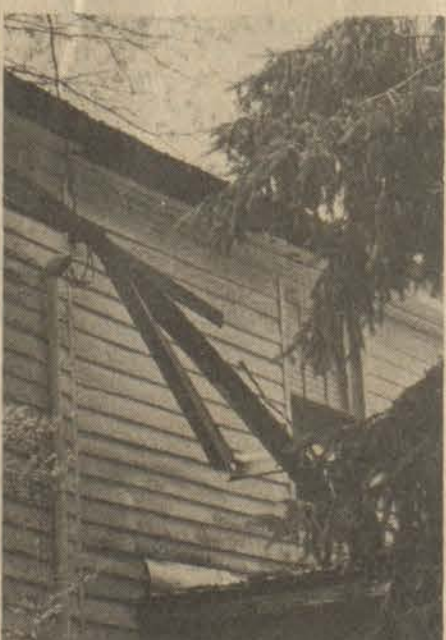
Water damage, largely the result of fallen gutters and downspouts, is taking its toll on the landmark.
