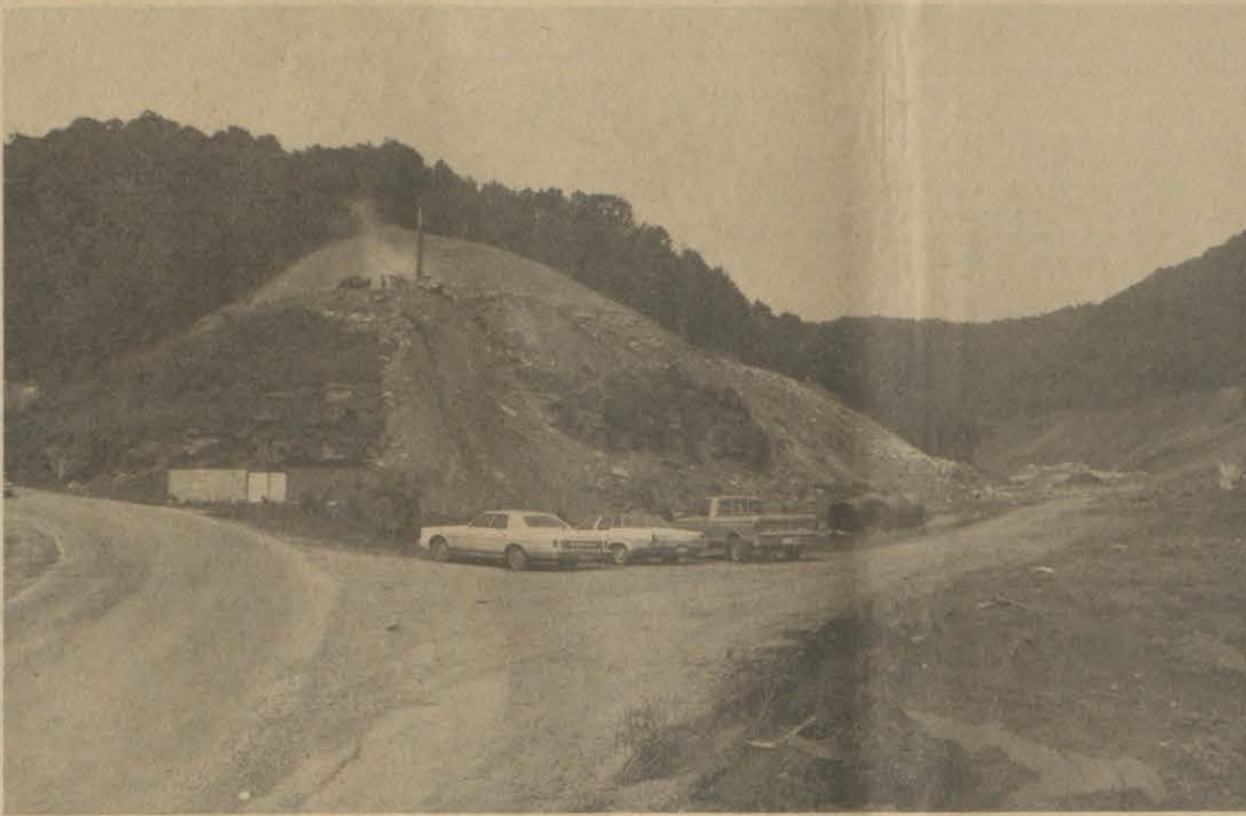
"Garrett Hollow," once filled with miners' homes built in the heyday of the Elk Horn Coal Corporation's mining activities at Garrett, is now cleared of every building of any size for the four-lane KY 80 under construction. Blasting is being done on the point running down onto old KY 80 to make room for four lanes of traffic. Across the old road (at left, out of camera range) work is under way on a four-lane bridge across Right Beaver Creek.
