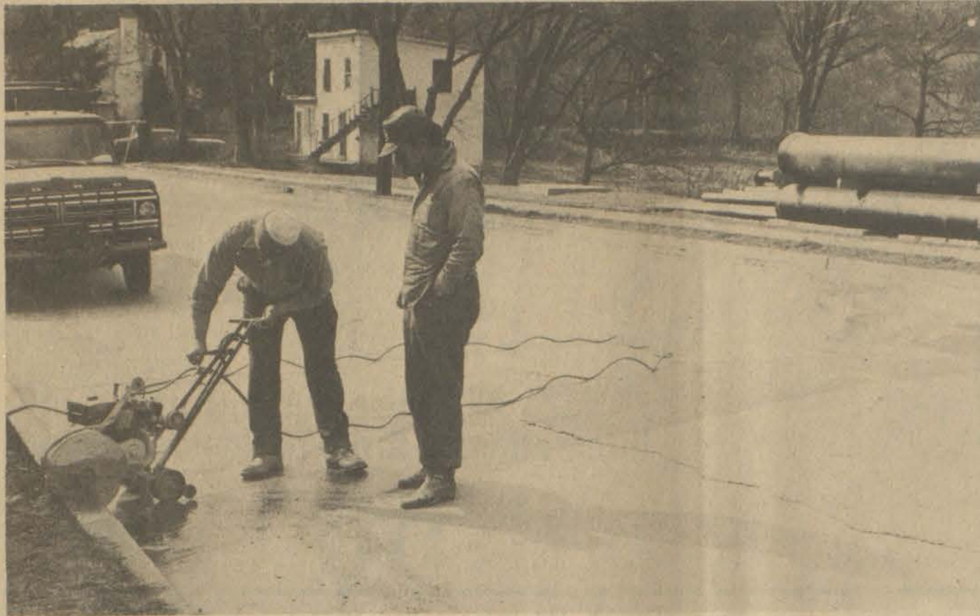
Workmen cut pavement across top of Prestonsburg floodwall in preparation for installation of new pump.
