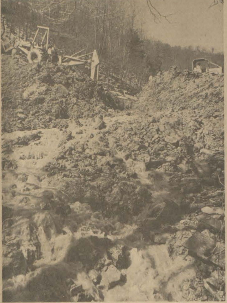
Water pours through a breach in the dike of the David reservoir as heavy equipment works at completion of drainage of the 4 1/2-acre impoundment. The reservoir, for years the water source for the community of David, was drained over the week-end in response to a recommendation by the Environmental Protection Agency (EPA) that drainage be done before spring rains create added stress to the dike which was declared by EPA to be unsafe.
