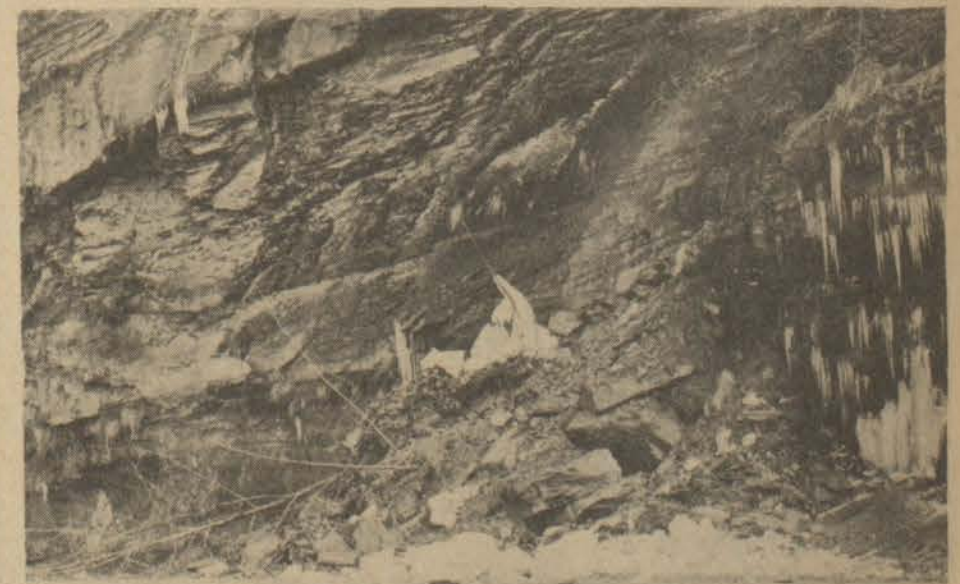
One very predictable result of the winter's sub-normal temperatures and heavy precipitation is an increased frequency of rock slides along US 23 between Prestonsburg and Paintsville. The slide pictured above on the Auxier Road is one of several which may be seen below the bordering cliffs on the route and as temperatures become warmer the slides are sure to become even more common. Repeated requests for state help in alleviating the problem have yet to bring results.
