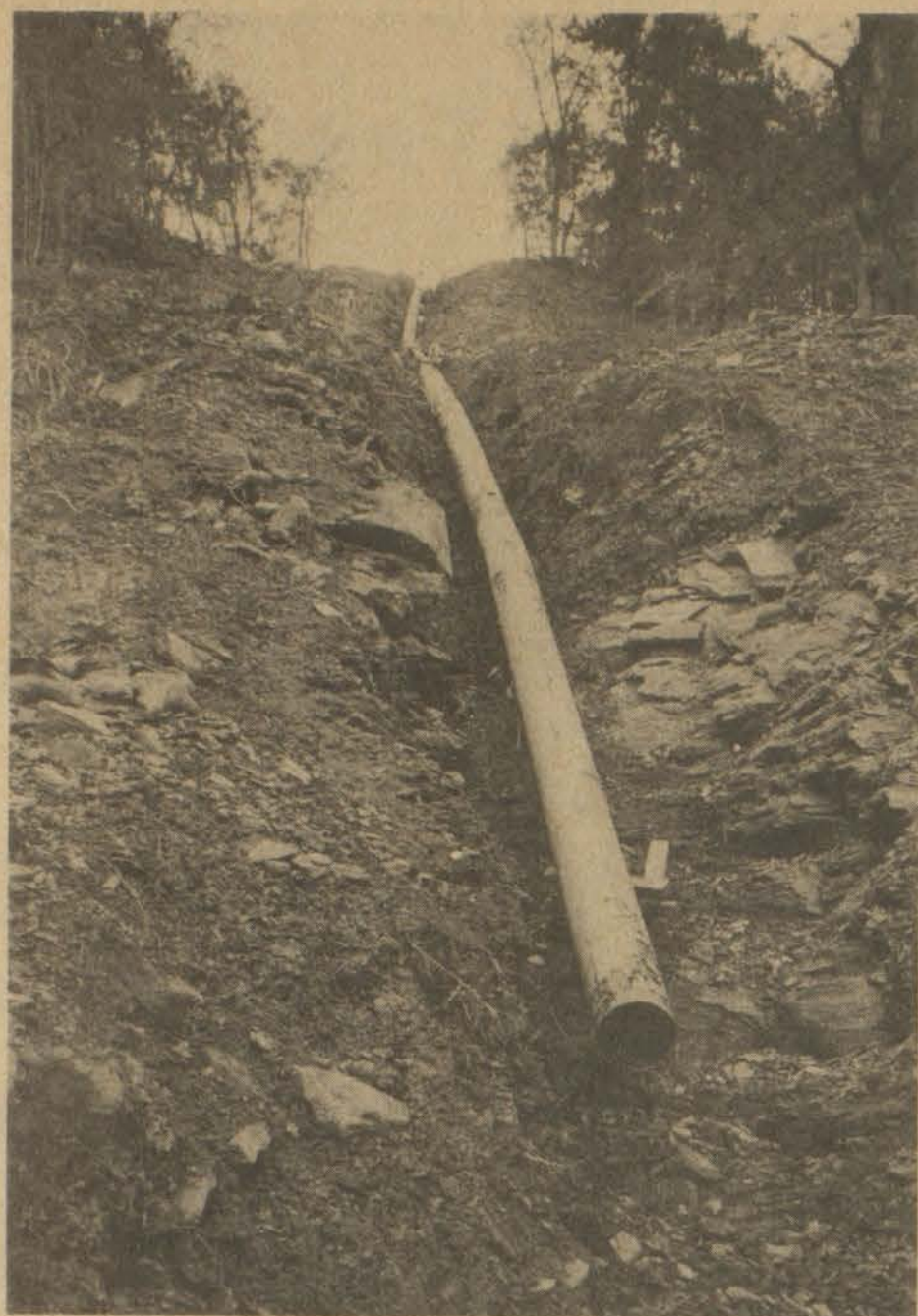
Relocation of pipeline to make way for construction of new KY 80 is occupying gas companies all along the designated route of the highway. Miles of pipeline are in the process of being moved or replaced in the Bull Creek-Water Gap area, the northern terminus of the new route. Columbia Gas Co. pipeline, such as the 20-inch line pictured above on the Right Fork of Bull Creek, is being rerouted over steep hills to avoid the path of Route 80.
