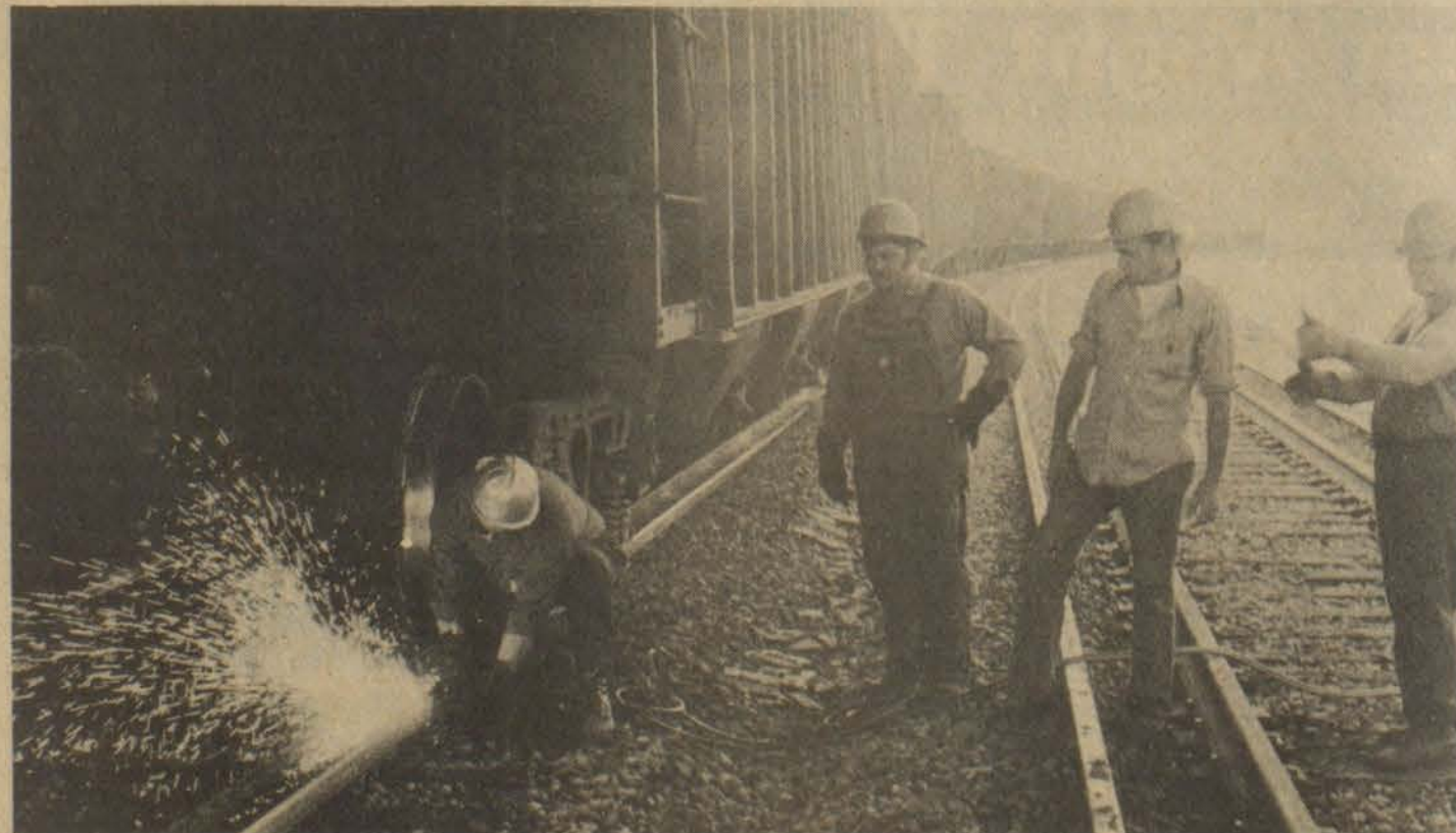
Workmen repair tracks at Dwale Thursday morning where 15 cars of a C. & O. train derailed at about 8 p.m. Wednesday. None of the loaded coal gondolas overturned and the track was returned to service by the week-end.
