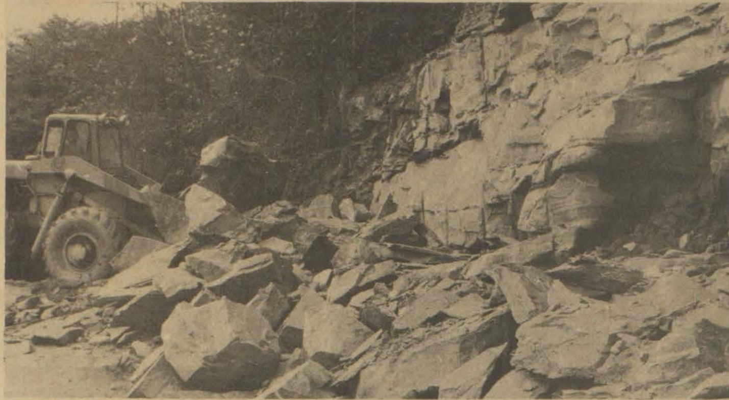
State Highway Department crews were at work this week widening a section of KY 404 (the David road) which has been plagued by repeated slips along the right-of-way. Photo shows excavation work on cliffside which will precede blacktopping of the broadened road surface.
