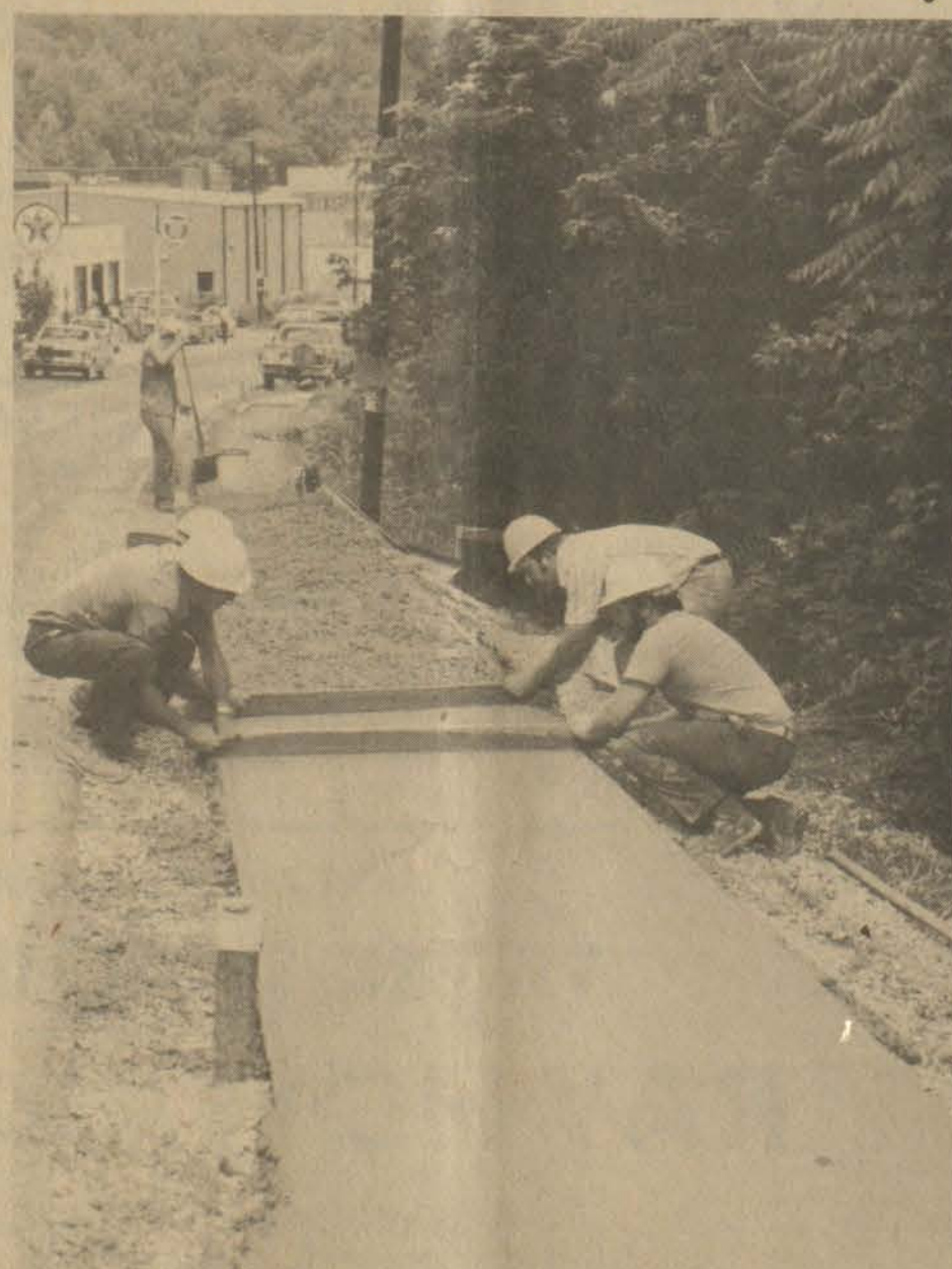
Concrete work at Martin which is presently under way will provide for about three-tenths mile of sidewalk in the lower end of the town near Martin Elementary. Utilizing state funds, the $15,000 project is designed primarily for the benefit of school children who must walk by the road side coming to and from school, it was said.
