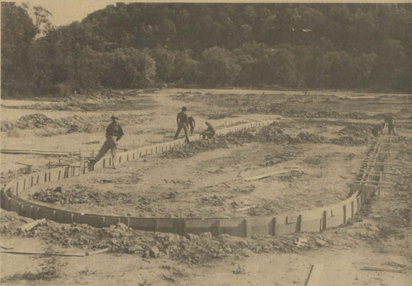
WORKMEN ARE PICTURED making preparations for the paving of a parking lot turnaround area to serve the new county park which has been under construction on the site of the Allen golf course since mid-March. Elmer Rice (pictured in foreground), project inspector for the county, said Phase I of the $1.5 million project is approximately 40 per cent complete. Contractor on the Phase I work is Big Wheel, Inc., of Angier, North Carolina.
