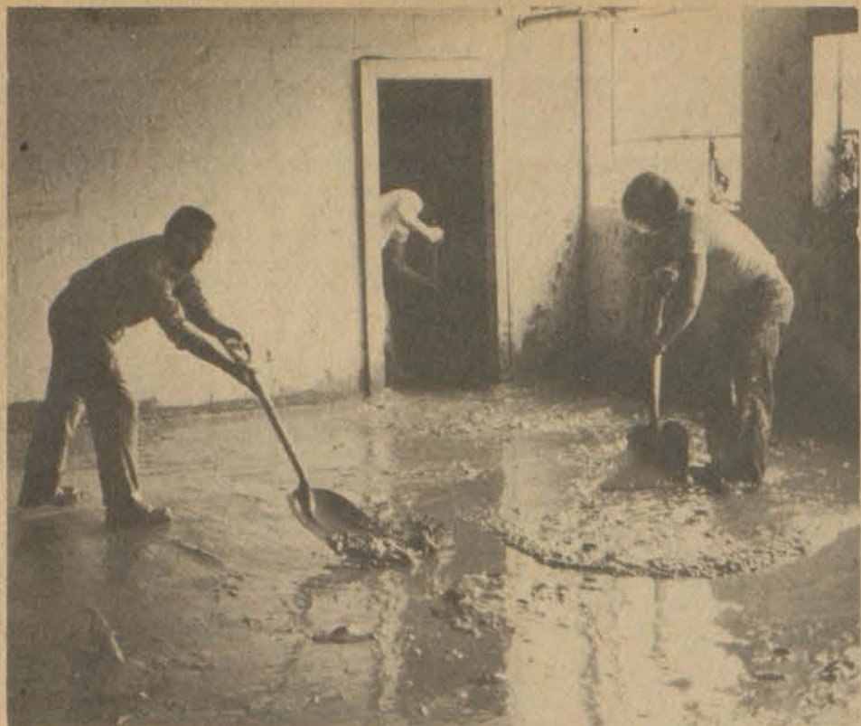
THREE INMATES from the Frankfort Career Development Center shovel mud from the basement of the Mullins school, near Pikeville. The men are part of a 25-man crew detached to Pikeville by the Bureau of Corrections to aid the community's recovery efforts following massive flood damage. An additional 25 men from the Blackburn Correctional Complex, near Lexington, have also been detached to the Pike county area this week, Corrections Commissioner David Bland has announced.
