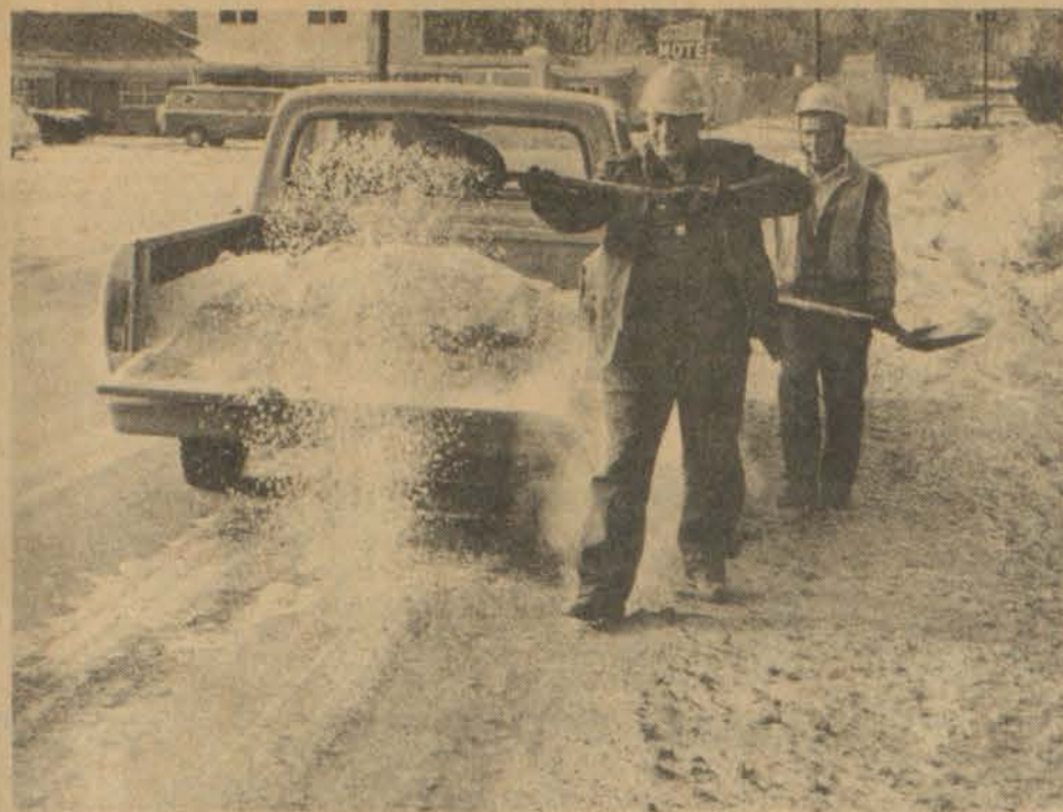
STATE HIGHWAY DEPARTMENT crews have been busy the past few weeks in an effort to keep area roads passable. In photo, workers distribute road salt, which has become a scarce commodity over the state, on an icy section of South Lake Drive here.
