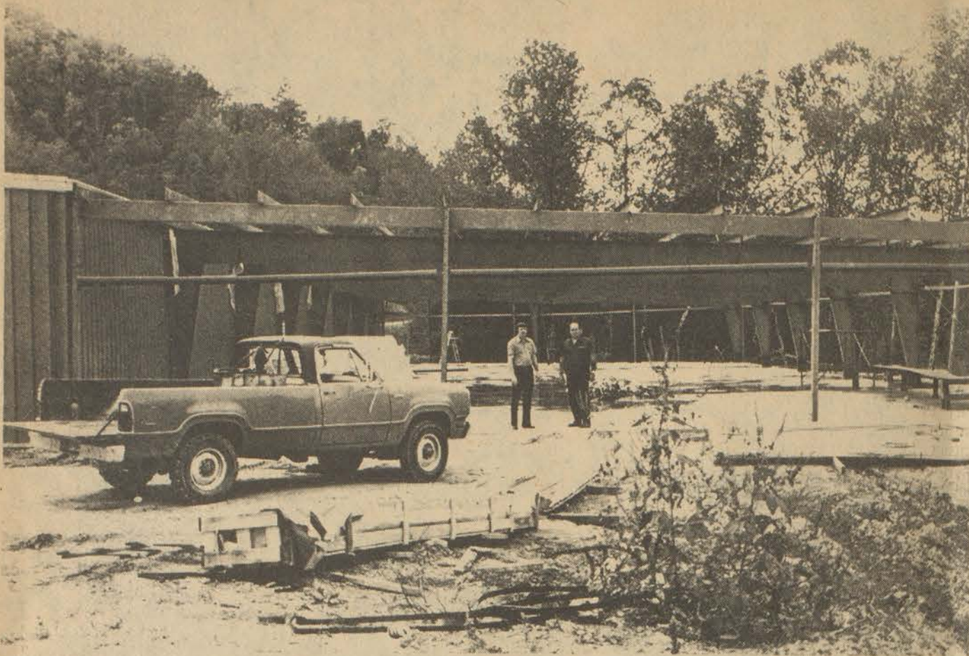
S-Mart, opened barely a year-and-a-half ago at Martin, is already enlarging to accomodate new lines of merchandise. The new addition will provide 10,500 more square feet to the building for a total of 30,500 sq. ft. The pre-fabricated metal addition is expected to be complete by November 15. S-Mart Manager Sam Hicks (at left) and owner of the building George Barnett are pictured at the site of the work.
