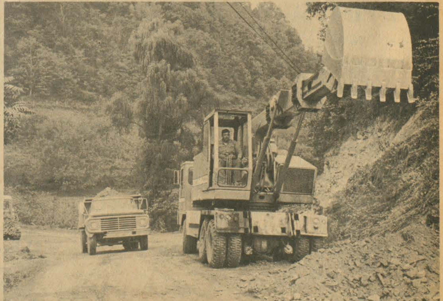
Highway Department workmen pictured providing fill dirt which is being used to elevate a flood-prone section of the Abbott Creek road at the mouth of Short Branch. Another low-lying section of the road has already been raised and the work, which was initiated through the efforts of the Abbott Creek Community Development Club, is expected to render the heavily travelled road passable through all but the most serious flooding.
