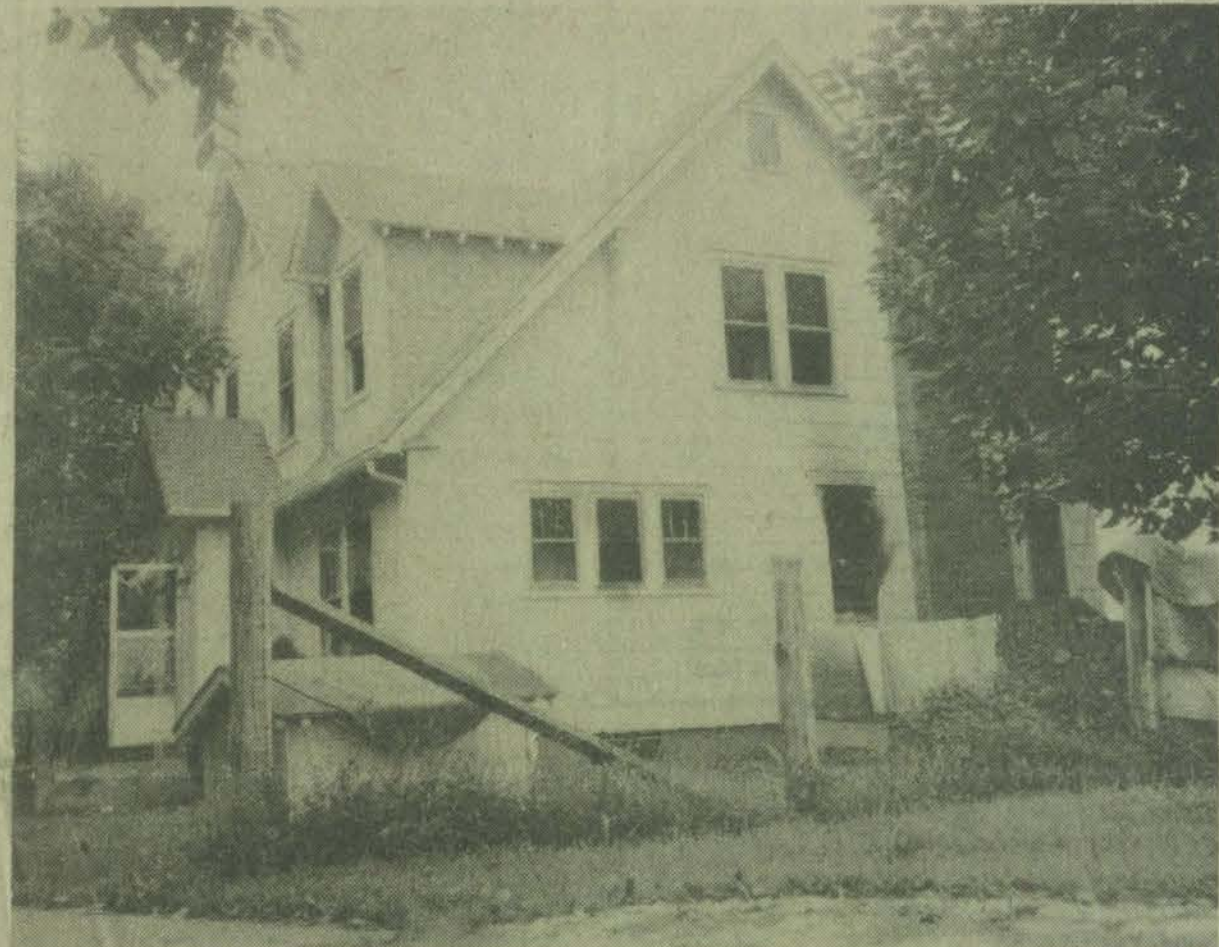
Exterior of Layne home shows only blackened area around a window near the location of a switch-box inside the house. Interior photo shows "melted" refrigerator, stove, other items.
