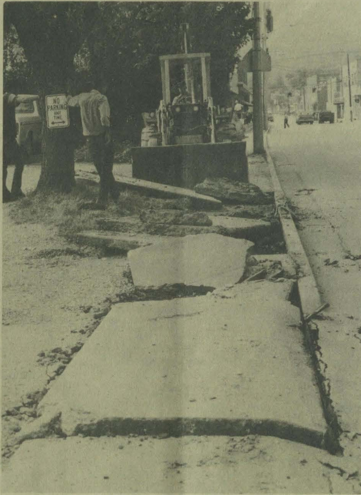
Workmen began breaking up the old walk along Lake Drive here this week, preparatory to new sidewalk construction.
