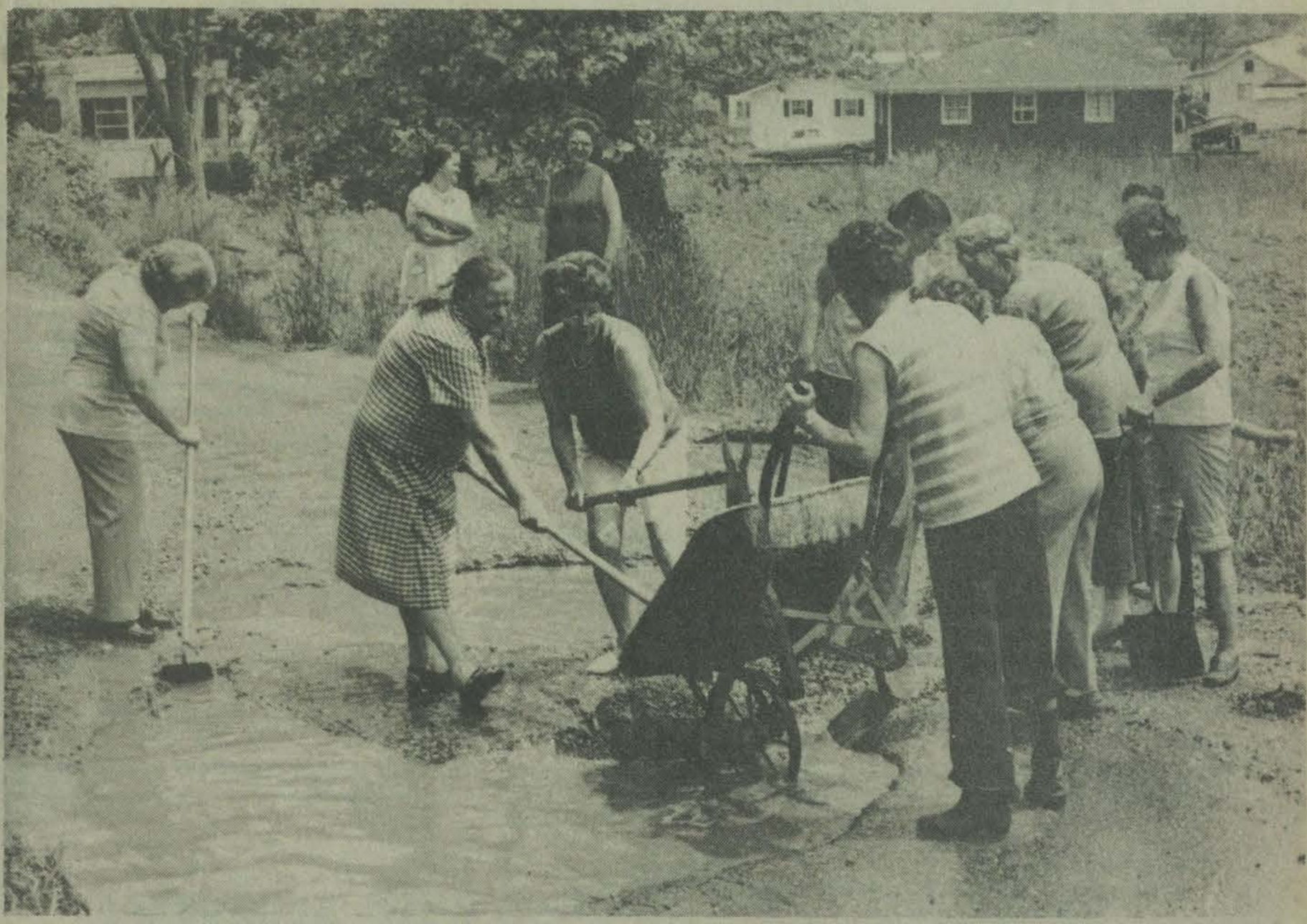
After repeated requests to the state highway department for road improvements had reportedly failed, this group of Dwale women decided last week to make certain improvements themselves—even without the use of road equipment. According to the women, the road, which is the approach to Dwale from new U.S. 23, has steadily deteriorated since the construction of new U.S. 23 a little over a year ago and caused serious drainage problems. The work involved ditching and draining the road and filling the ruts with rocks which they carried some distance.
