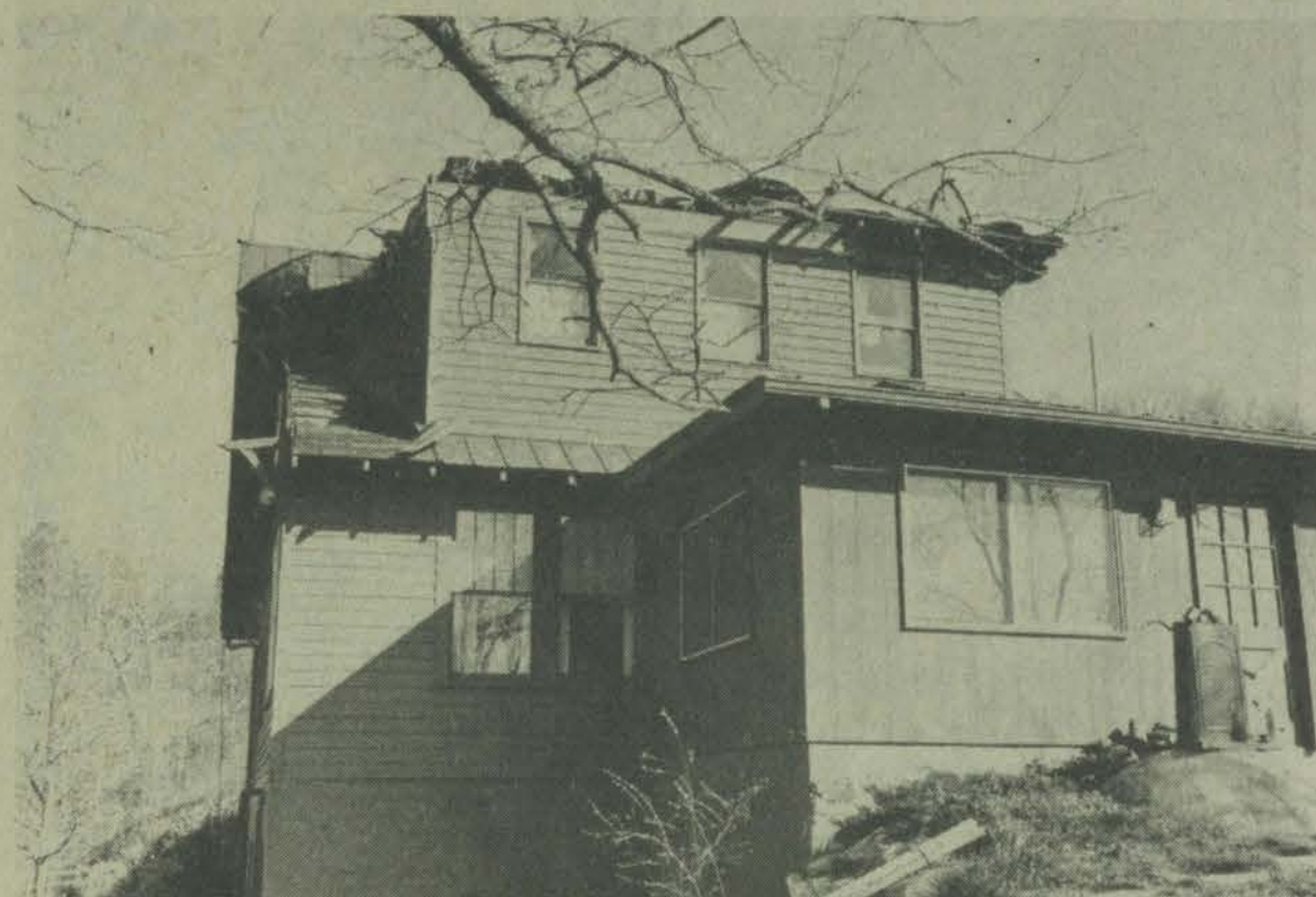
Front view of the Harris Howard home, showing a portion of the roof damage.
