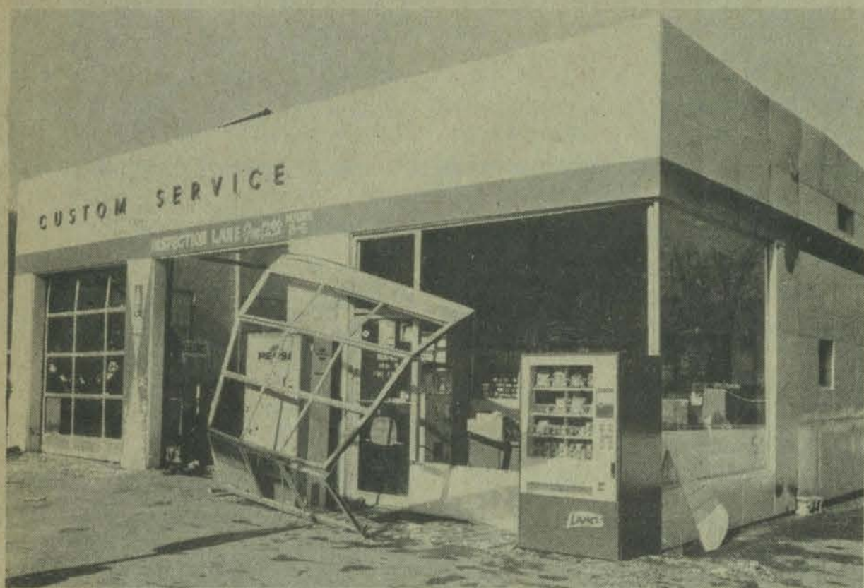
Front view of Compton's Phillips 66 Station here shows broken glass and twisted door but fails to picture ruined roof after windstorm.
