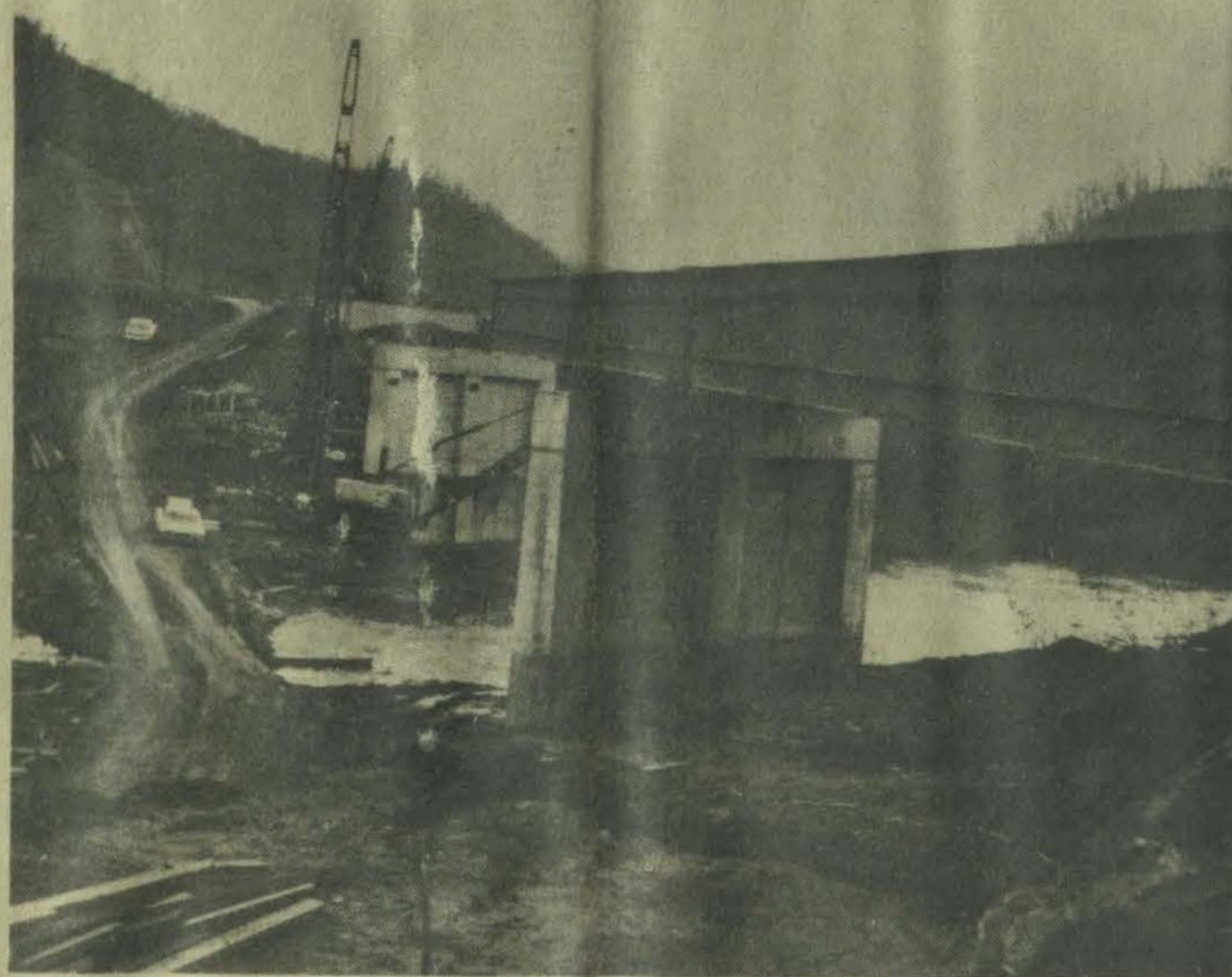
SHAPING UP. Photo shows progress being made on bridge spanning the Big Sandy at Lancer and connecting old US 23 with the Bull Creek road now under construction. The span will be one of the more heavily travelled in the area, since it will carry traffic from the yet-to-be-built US 23 at Water Gap to the Prestonsburg area and Jenny Wiley State Park as well as serve the Goble-Roberts Addition and the U. S. Shoe Company plant there.
