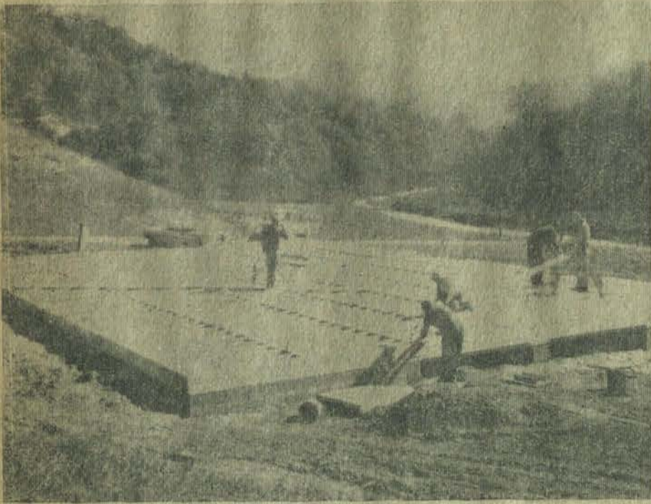
Floyd County Fish & Game Club members are losing no time getting their clubhouse going up in the Johns Branch valley, near Maytown. Groundbreaking ceremonies were held Sept. 1, and with clubmembers donating their work the foundation and subfloor have been completed. They hope to have the structure under roof before winter weather arrives and to have it ready for use next spring.
